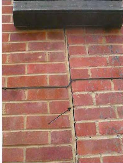
Crack at junction of extension on right side.
