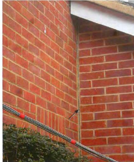
Cracking at junction of extension on left side.
