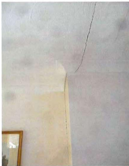
Cracking at extension junction in hall.
