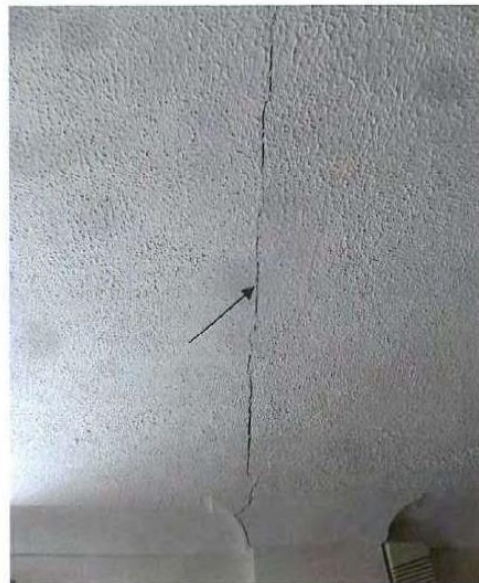
Crack at extension junction in bedroom.
