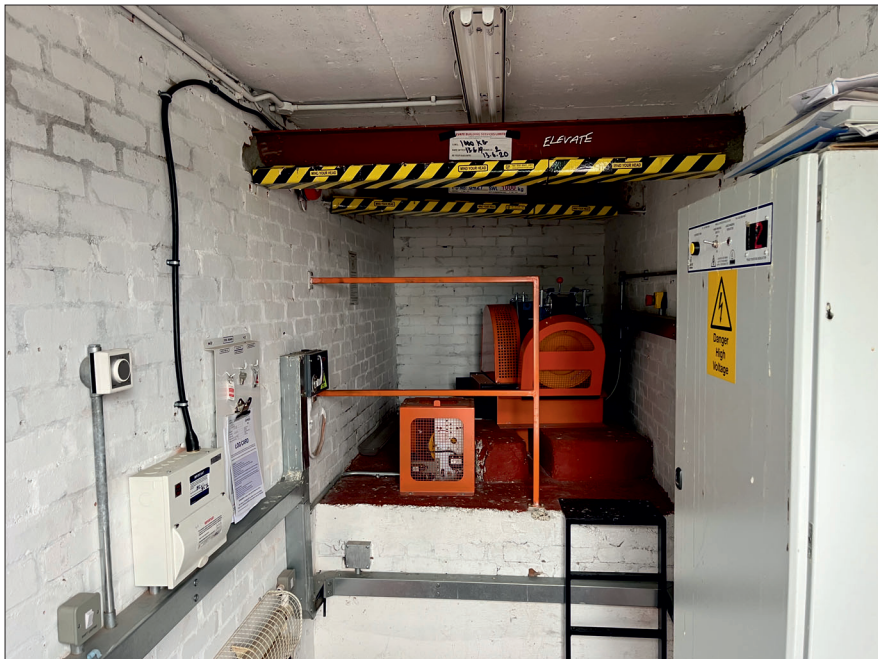
Photograph 4: Showing the inside of the service unit, housing the lift mechanism.
