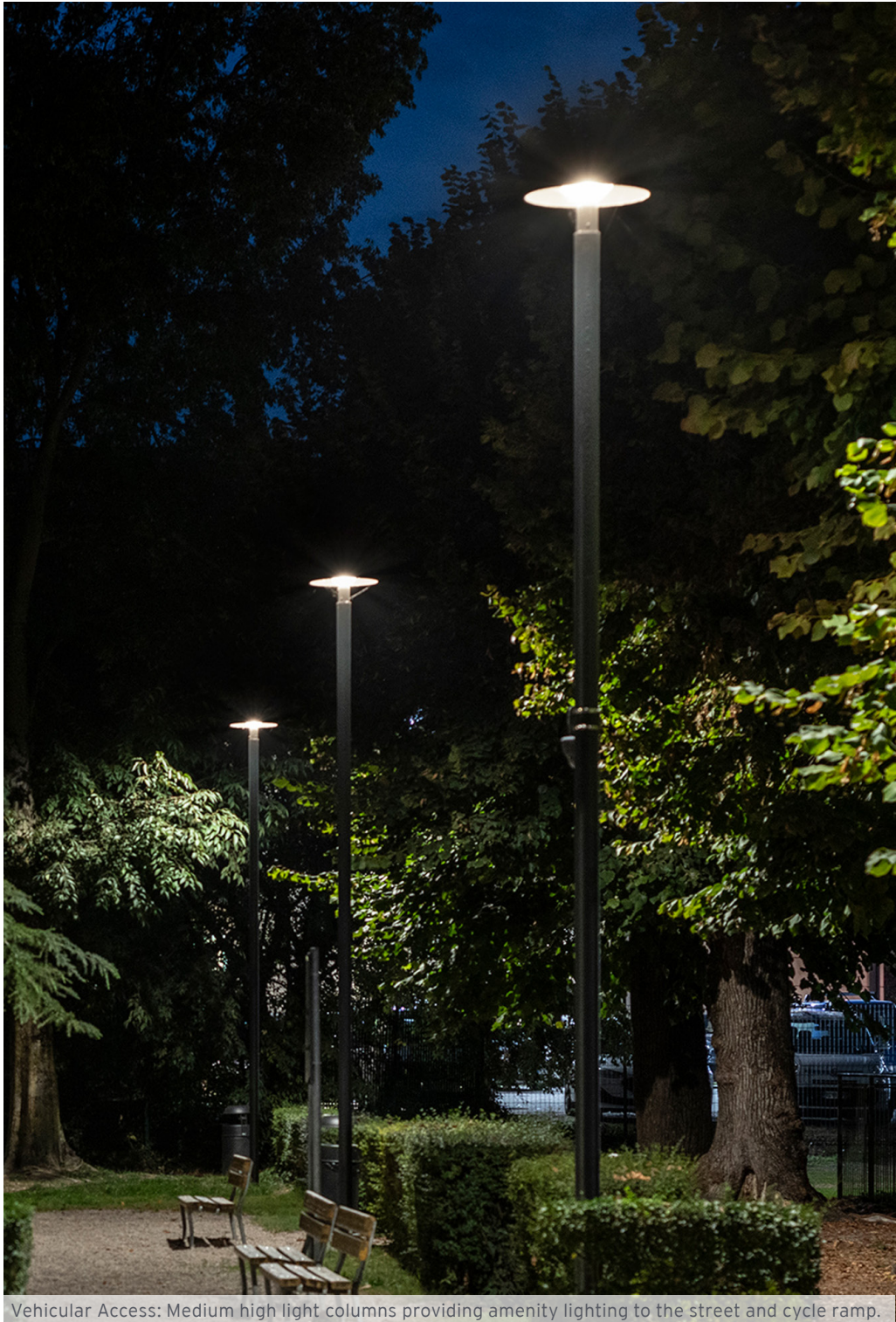
Vehicular Access: Medium high light columns providing amenity lighting to the street and cycle ramp.
