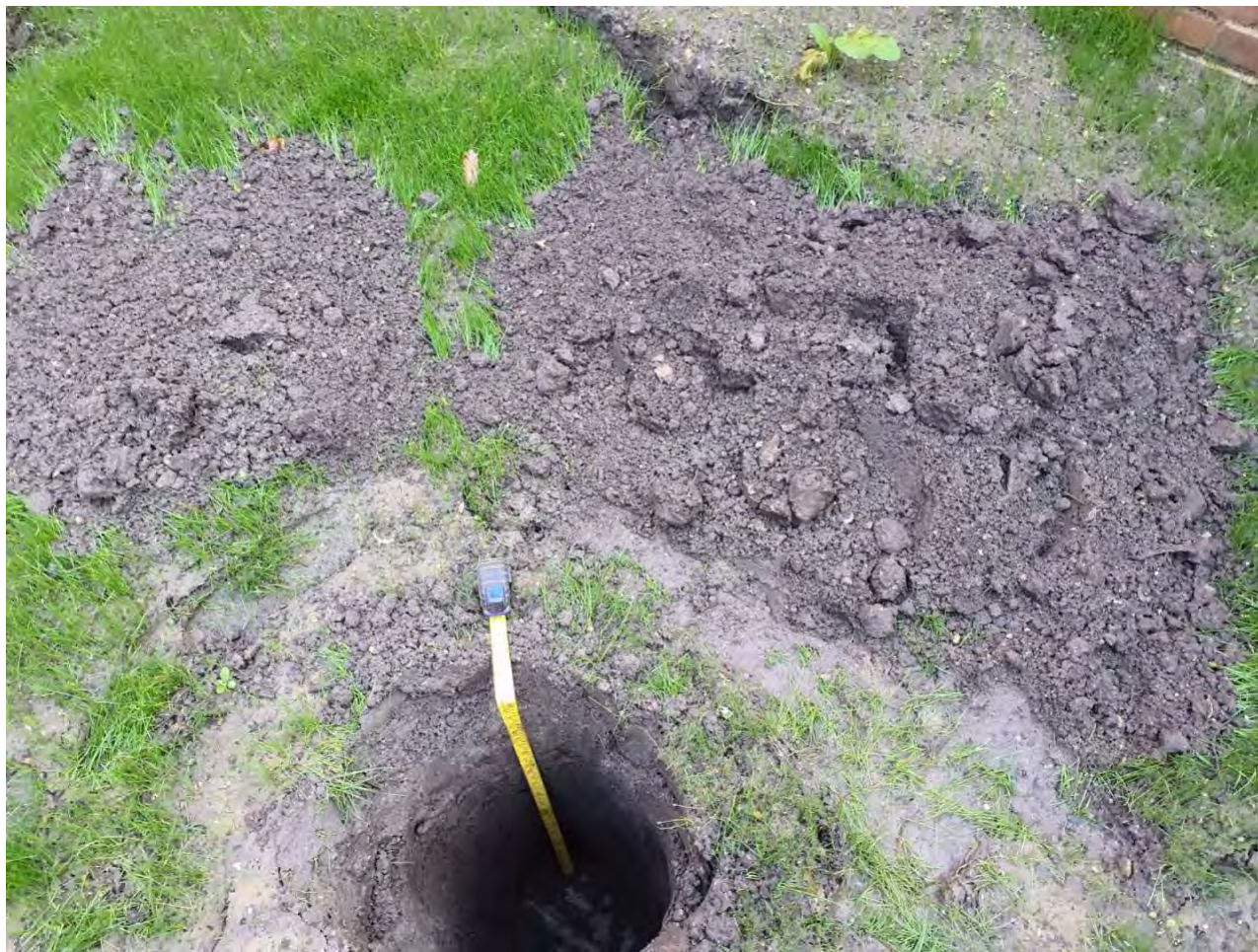
Photo of hole with tape in place
