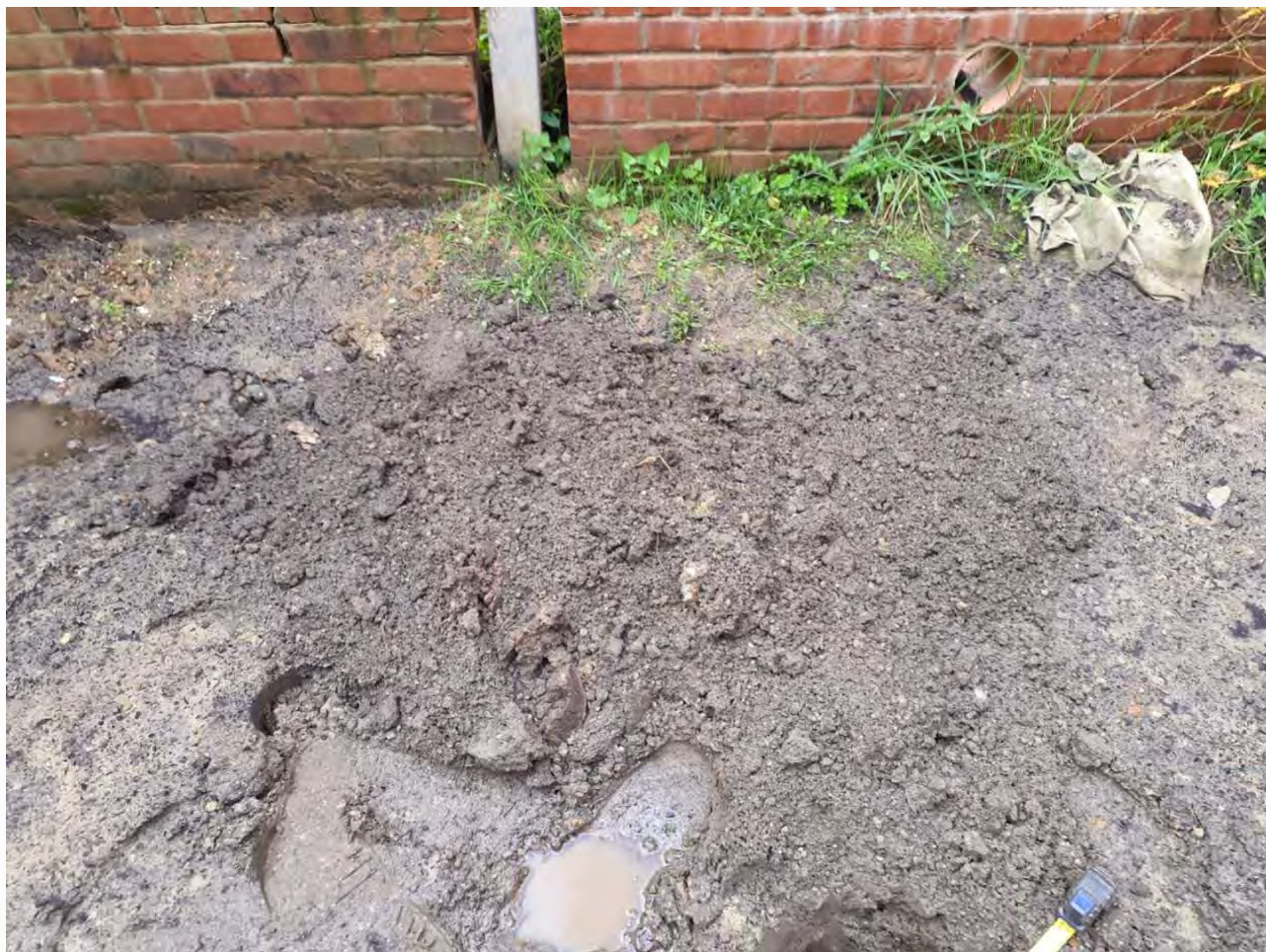
Photo of hole with tape in place
