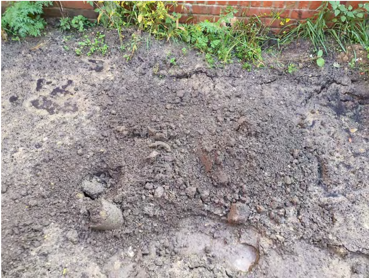
Photo of hole with tape in place
