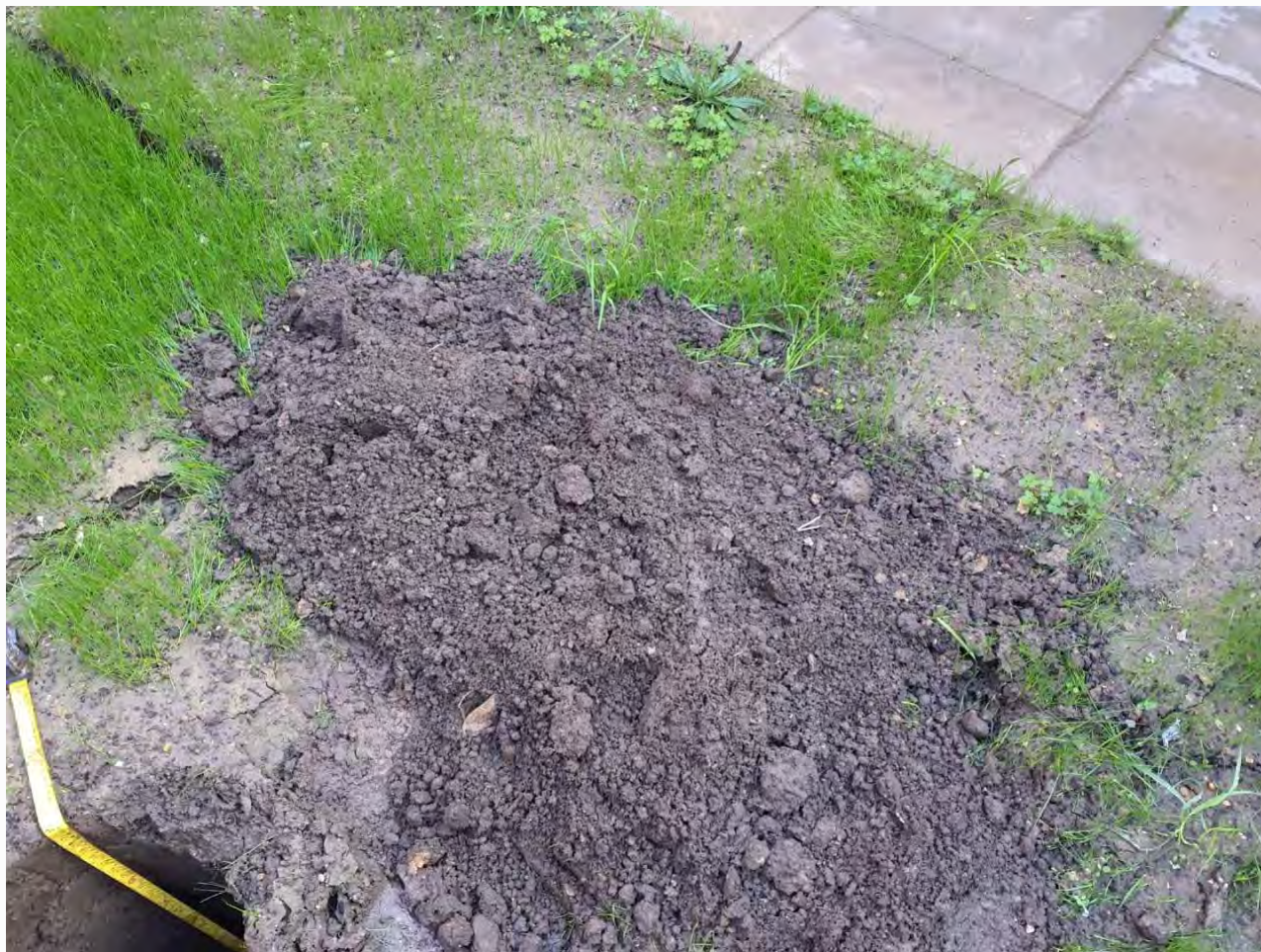
Photo of hole with tape in place
