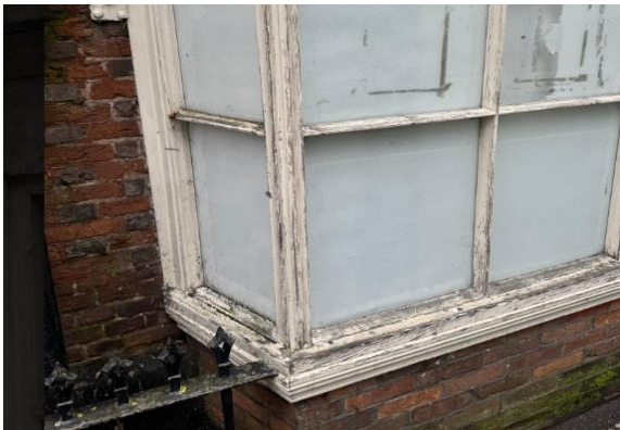
Fig. 14: Detail of the left-hand shopfront window, with condition of paintwork.
