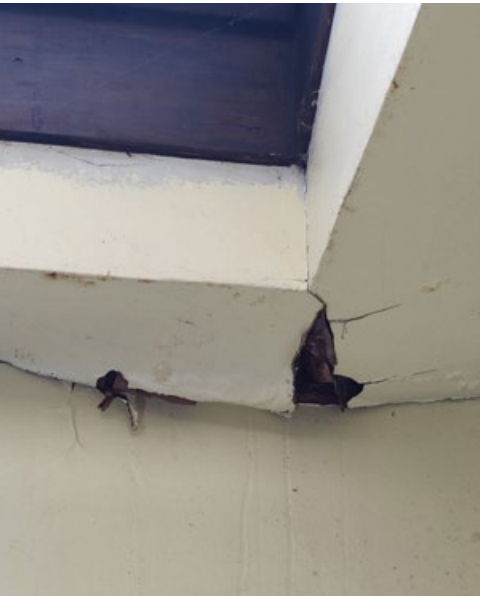
Level 1 bathroom ceiling water damage
