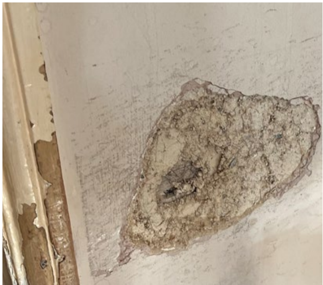
Damage to original lime plaster
