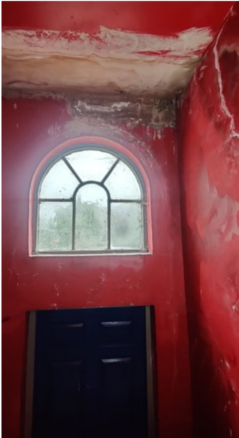
GF hallway ceiling water damage
