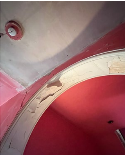
GF hallway ceiling water damage
