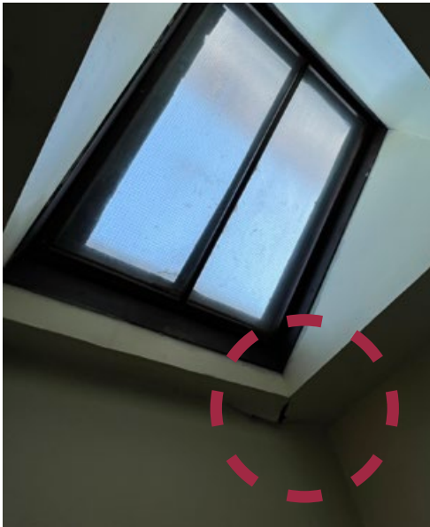
Level 1 bathroom ceiling water damage
