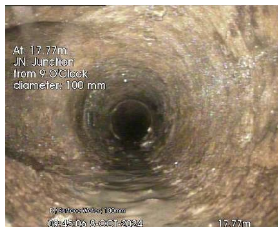
SW1 DOWNSTREAM INTERCEPTOR_17-77m_094506.jpg, 00:03:25, 17.77 m Junction at 9 o'clock, 100mm dia
