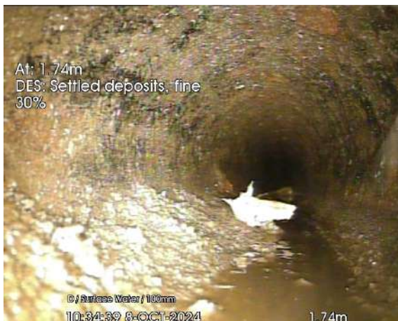
SW2 DOWNSTREAM INTERCEPTOR_1-74m_103439.jpg, 00:00:44, 1.74 m Settled deposits, fine, 30% cross-sectional area loss
