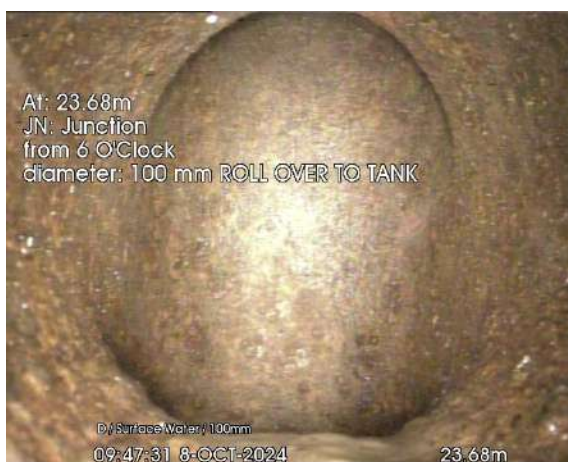
SW1 DOWNSTREAM INTERCEPTOR_23-68m_094731.jpg, 00:04:45, 23.68 m Junction at 6 o'clock, 100mm dia, ROLL OVER TO TANK
