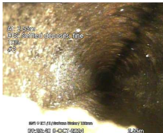
SW1 UPSTREAM IC1_2-55m_092540.jpg, 00:00:57, 2.55 m Settled deposits, fine, 10% cross-sectional area loss, start
