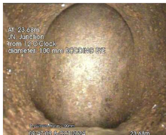
SW1 DOWNSTREAM INTERCEPTOR_23-68m_094709.jpg, 00:04:41, 23.68 m Junction at 12 o'clock, 100mm dia, RODDING EYE
