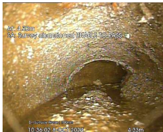
SW2 DOWNSTREAM INTERCEPTOR_4-33m_103602.jpg, 00:01:34, 4.33 m Survey abandoned, UNABLE TO PASS
