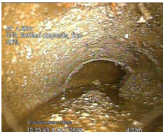
SW2 DOWNSTREAM INTERCEPTOR_4-33m_103543.jpg, 00:01:30, 4.33 m Settled deposits, fine, 60% cross-sectional area loss
