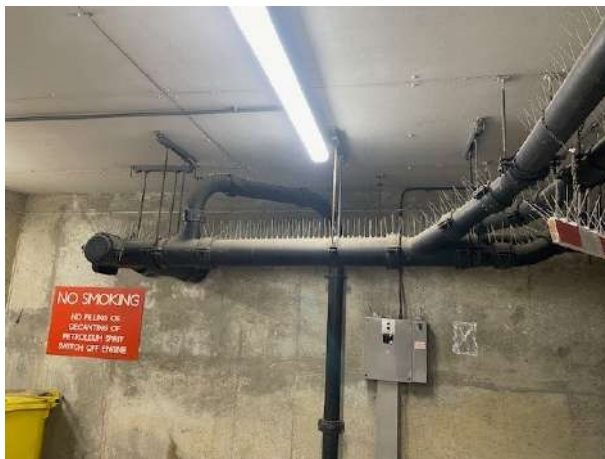
PUMP OUTLET TO MAINS IN ROAD
