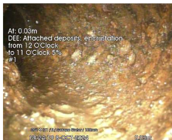
SW1 UPSTREAM IC1_0-03m_092419.jpg, 00:00:16, 0.03 m Attached deposits, encrustation from 12 o'clock to 11 o'clock, 5% cross-sectional area loss, start
