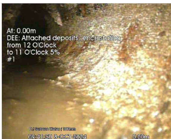
SW1 DOWNSTREAM INTERCEPTOR_0-00m_094150.jpg, 00:00:19, 0.00 m Attached deposits, encrustation from 12 o'clock to 11 o'clock, 5% cross-sectional area loss, start
