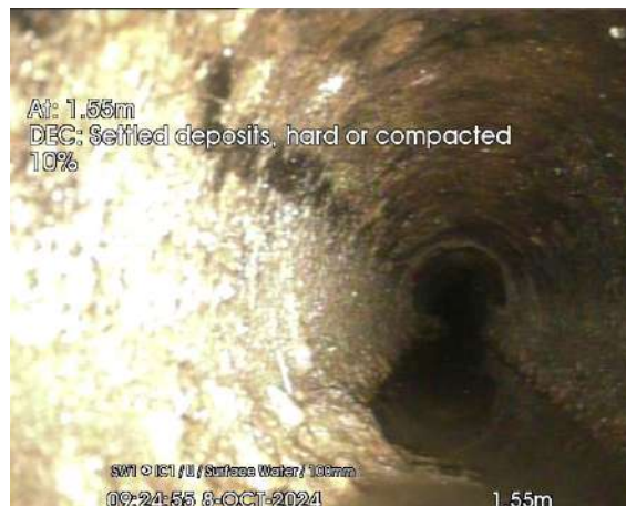
SW1 UPSTREAM IC1_1-55m_092455.jpg, 00:00:34, 1.55 m Settled deposits, hard or compacted, 10% cross-sectional area loss
