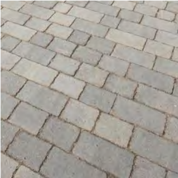
Permeable paving to reduce stormwater runoff volume
