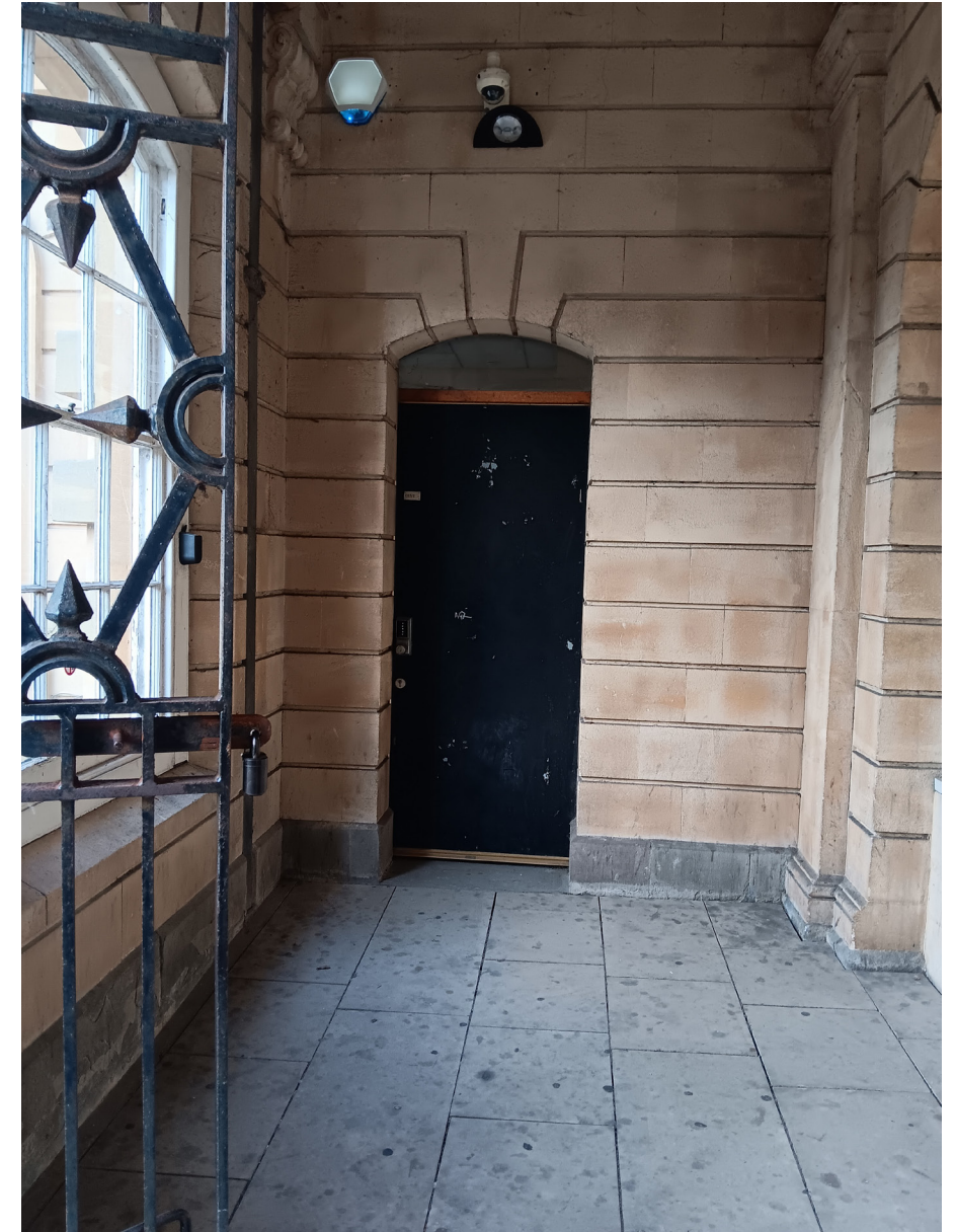
Fig.06 Existing door at restricted (north) entrance to be replaced..
