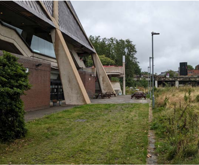
① Existing terraces need maintenance and are unclear how to access
