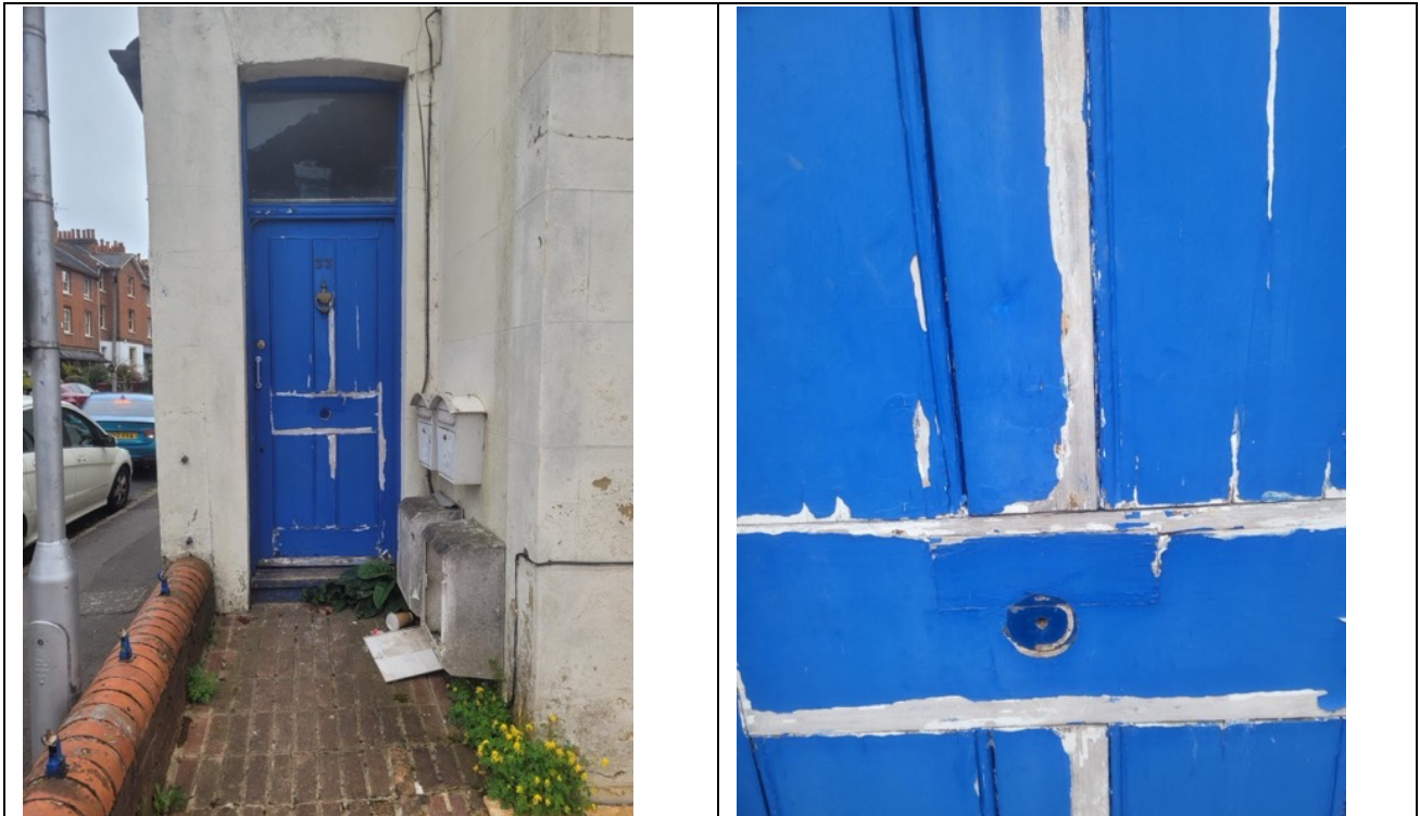
Figure 2 (Left) front door of 33 Baker Street and (Right) detail of front door and missing door knob
