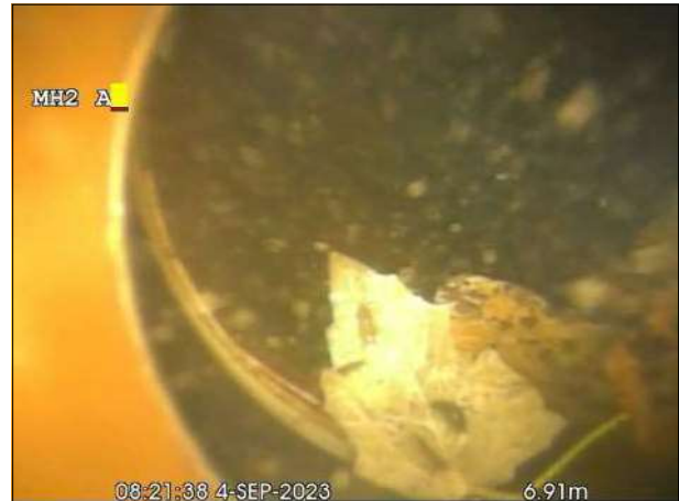
Photo: 33_6a, 00:00:00 7m, Joint displaced. Medium
