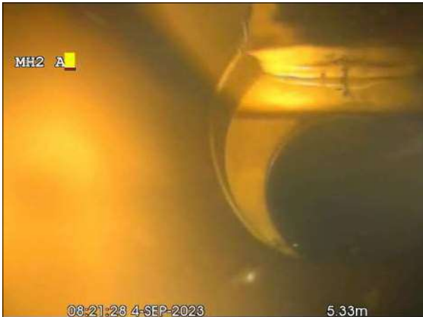
Photo: 32_5a, 00:00:00 5.6m, Dimension of sewer changes, new dimension dia 100 mm
