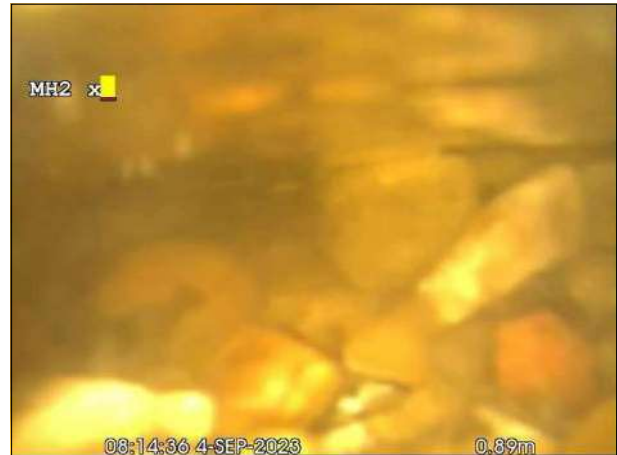
Photo: 1_5a, 00:00:00 0.89m, Debris, 20 % cross-sectional area loss
