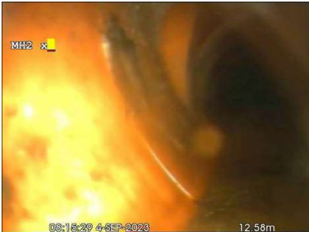
Photo: 17_14b, 00:00:00 12.6m, Junction at 10 o'clock, dia 100 mm
