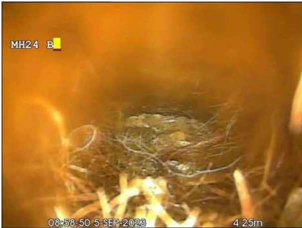
Photo: 344_5a, 00:00:00 4.9m, Debris, 95 % cross-sectional area loss
