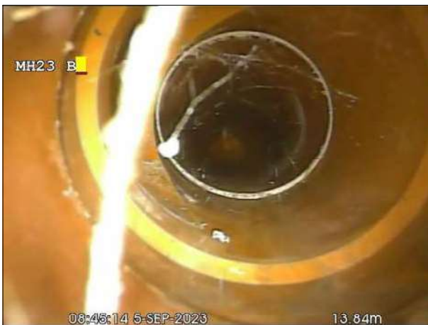
Photo: 323_7a, 00:00:00 13.8m, Joint displaced. Medium
