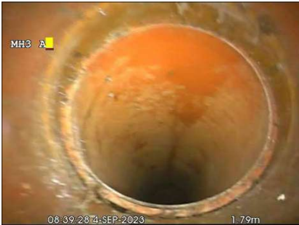
Photo: 70_5a, 00:00:00 1.8m, Joint displaced. Medium
