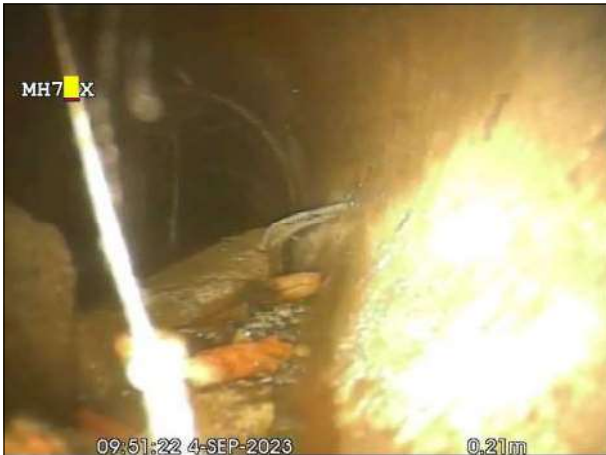
Photo: 15_3a, 00:00:00 0.3m, Debris, 30 % cross-sectional area loss
