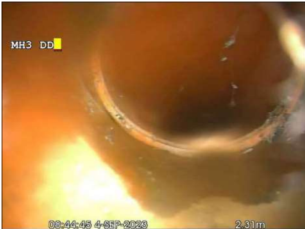
Photo: 8_6a, 00:00:00 2.5m, Joint displaced. Medium
