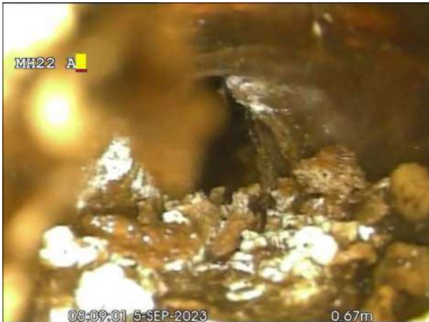
Photo: 278_5a, 00:00:00 0.7m, Debris, 50 % cross-sectional area loss
