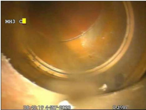
Photo: 84_3a, 00:00:00 0.4m, Joint displaced. Medium
