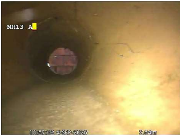
Photo: 187_4a, 00:00:00 2.5m, Circumferential Crack, from 12 to 01 o'clock
