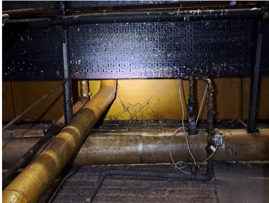
Photo 7. Showing a small gap between some metal services and the wall, covered by cobwebs and debris
