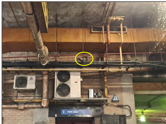
Photo 5. A gap in the brickwork, also cluttered by pipes and services in the eastern end of the service area.
