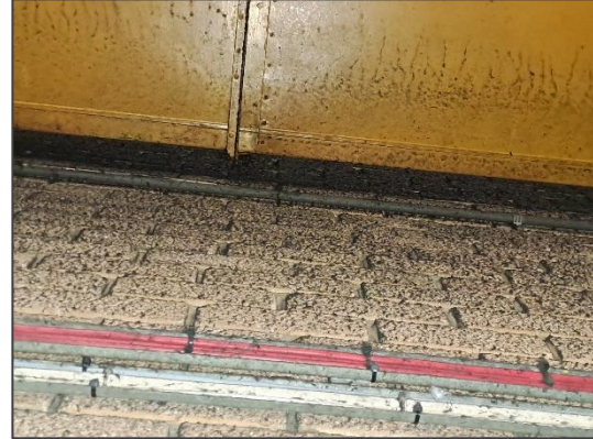
Photo 8. Showing the dirt and dust accumulated on the walls of the service area
