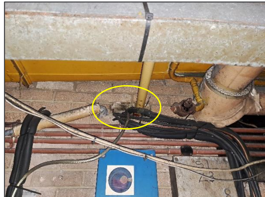
Photo 4. Showing a gap in the brickwork, cluttered by pipes and services
