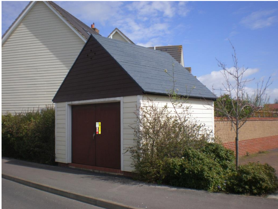
Photograph 1 -The photograph shows a typical installation with a removable roof. The outside brick has been clad to match the surrounding buildings. The doors are GRP.
