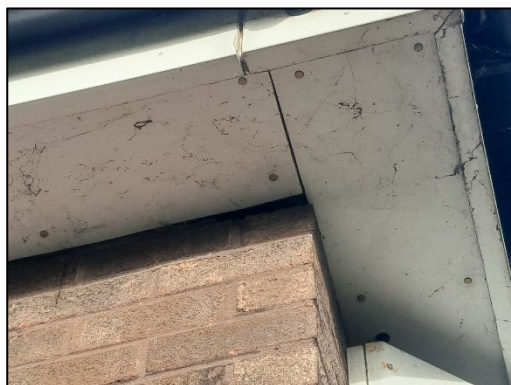
Figure 17: Gap behind soffit boxes on southern elevation of building.
