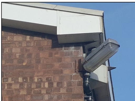
Figure 20: Gaps within and behind soffit boxes on building, creating potential access points for breeding birds.
