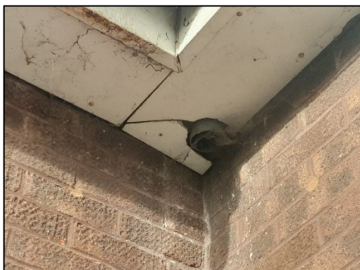
Figure 16: Cracks and gaps in soffit boxes on southern elevation of building.
