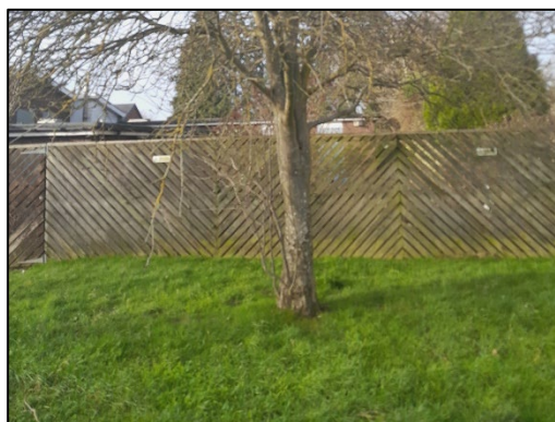
Figure 13: Wooden panel fence.
