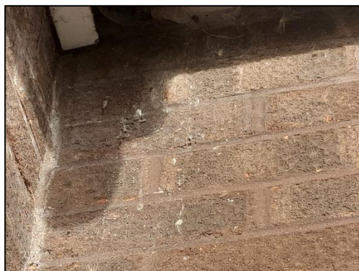
Figure 16: Bird faeces on brick walls of building.
