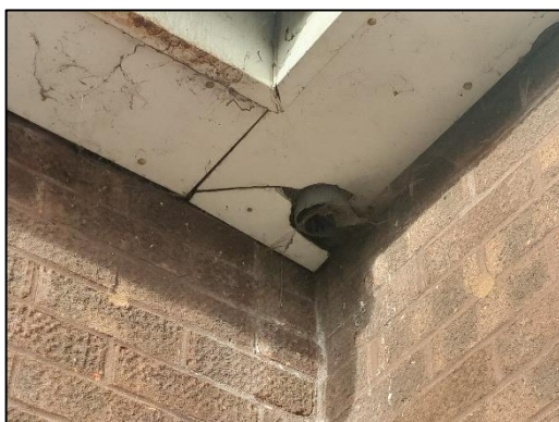
Figure 11: Cracks and gaps in soffit boxes on southern elevation of building.
