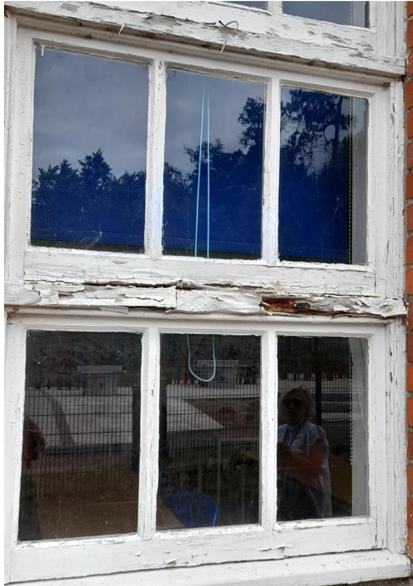
Fig. 17: Detail of ground-floor window of B Block, with evidence of advanced decay of window frames.
