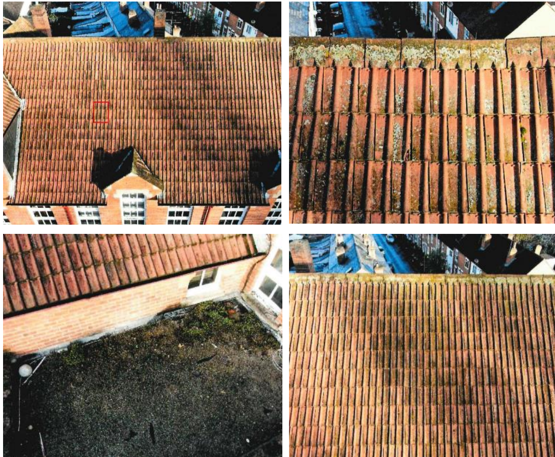
Fig. 18: Photographs of defective areas of tiled roof on B Block (St Joseph's College).
