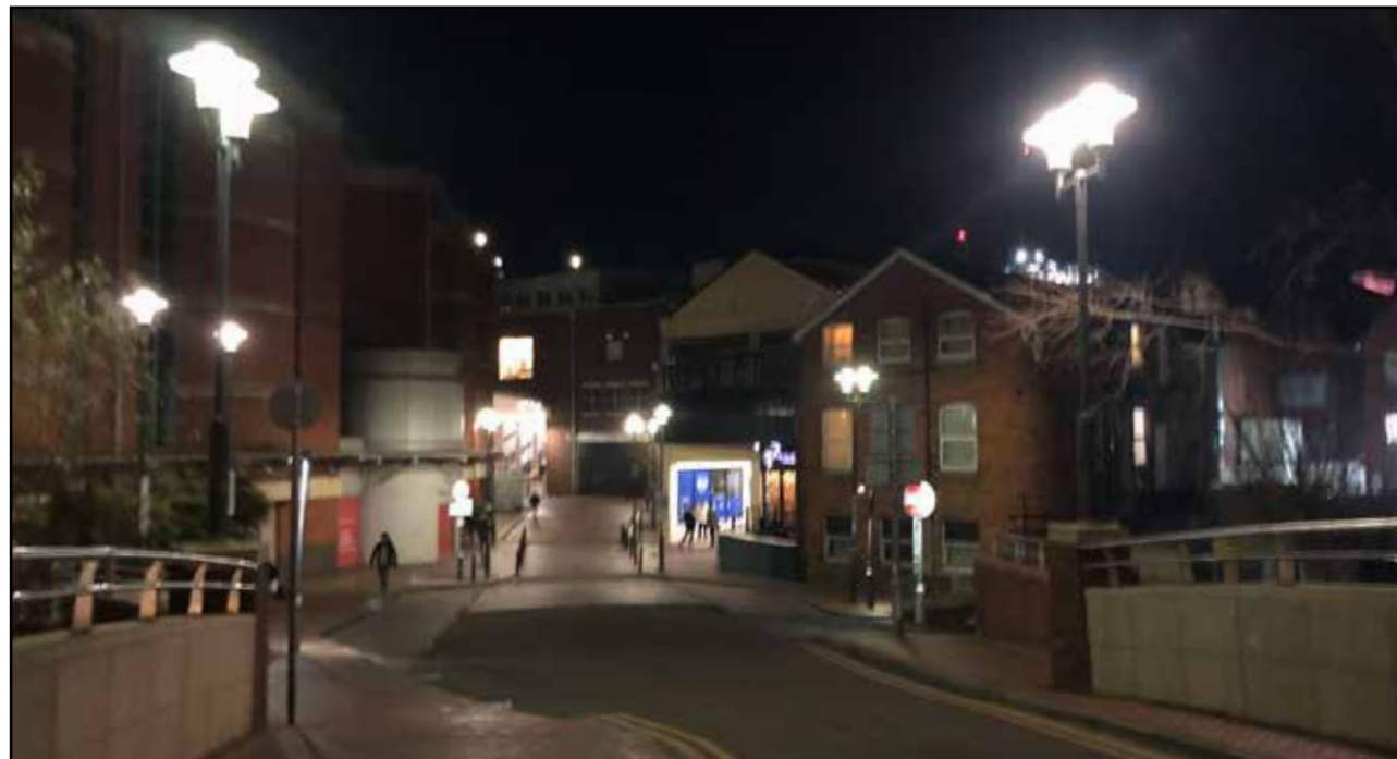
Figure 5.49 Showing LED luminaires mounted on approximately 6m high columns along Yield Hall Place, looking north-west. Captured at approximate position of Survey Location A1.
