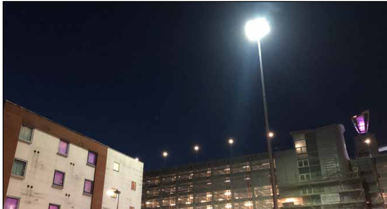
Figure 5.69 Showing luminaire mounted on 30 metre high column along A329/Mill Lane, looking north-west. MSCP in background. Captured at approximate position of Survey Location A19.
