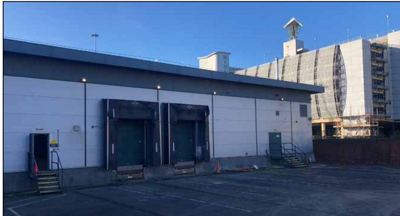
Figure 5.25 showing LED floodlights on building facade, facing west. Captured at approximate position of Survey Location A9.
