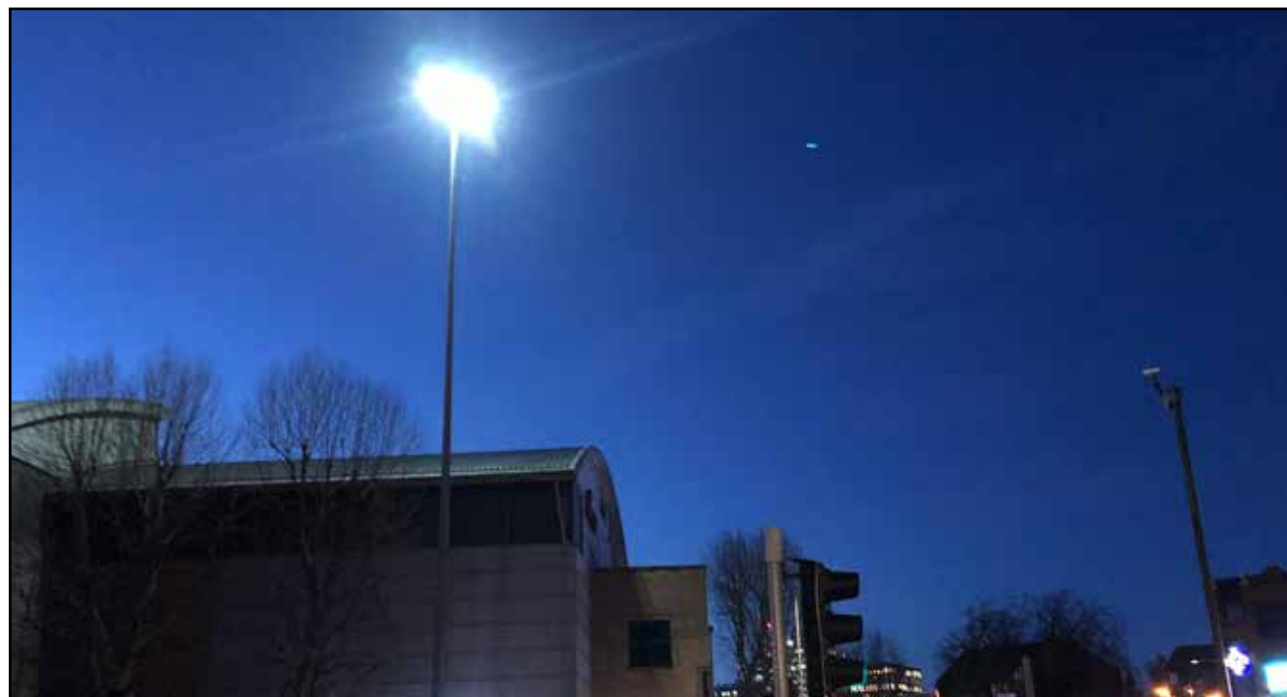
Figure 5.57 Showing luminaire mounted on 30 metre high column along A329/Mill Lane, looking north-west. Captured at approximate position of Survey Location A3.
