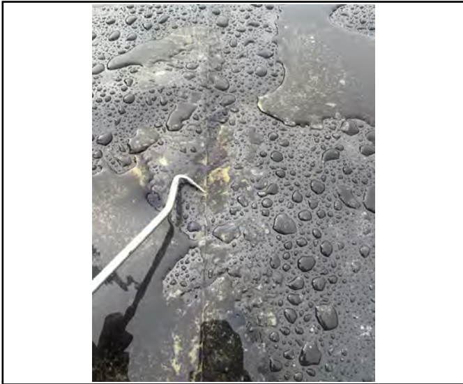
Pick and probe test conducted upon a sealed lap joint.
