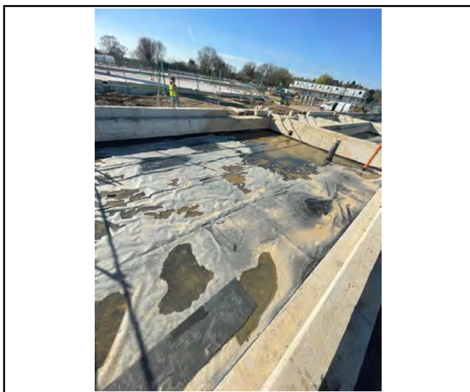
Outstanding remediations, remediated
