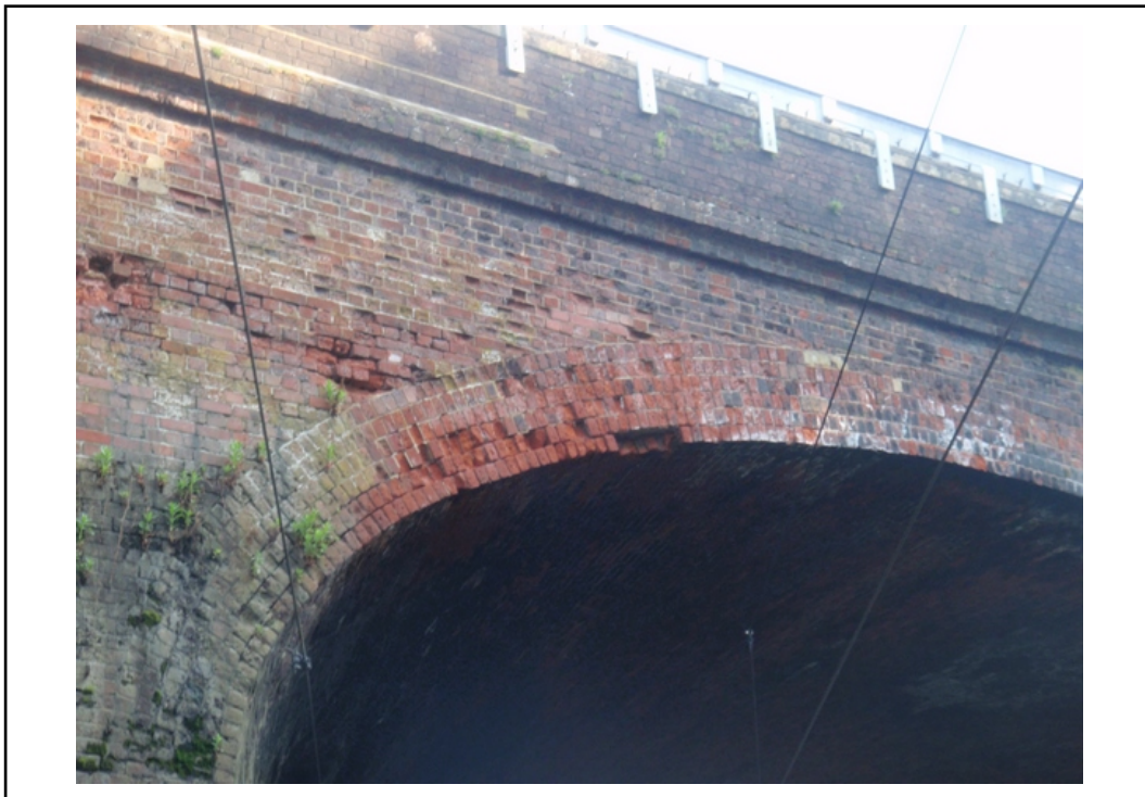
Photo No 6 - Showing missing brickwork to bottom ring 11/05/24 -
