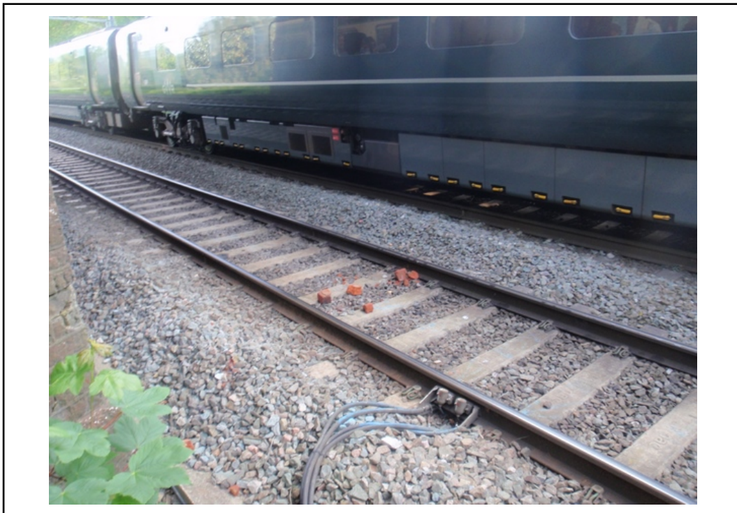
Photo No 8 - Showing fallen brickwork in the up Westbury line 11/05/24 -
