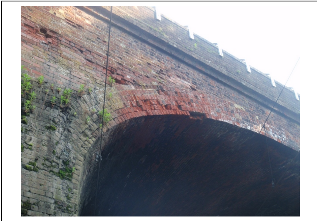
Photo No 7 - Showing missing brickwork to bottom ring 11/05/24 -
