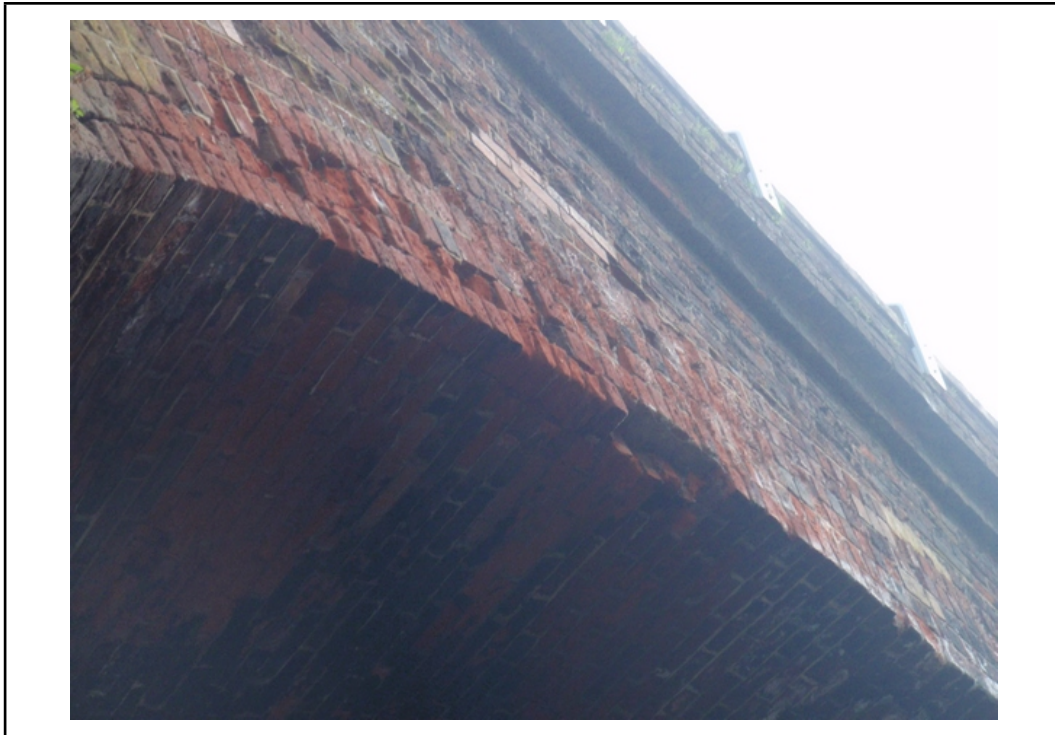
Photo No 5 - Showing missing brickwork to bottom ring 11/05/24 -
