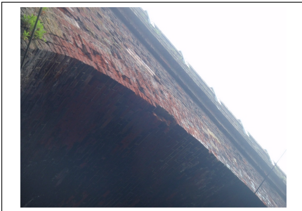
Photo No 4 - Showing missing brickwork to bottom ring 11/05/24 -
