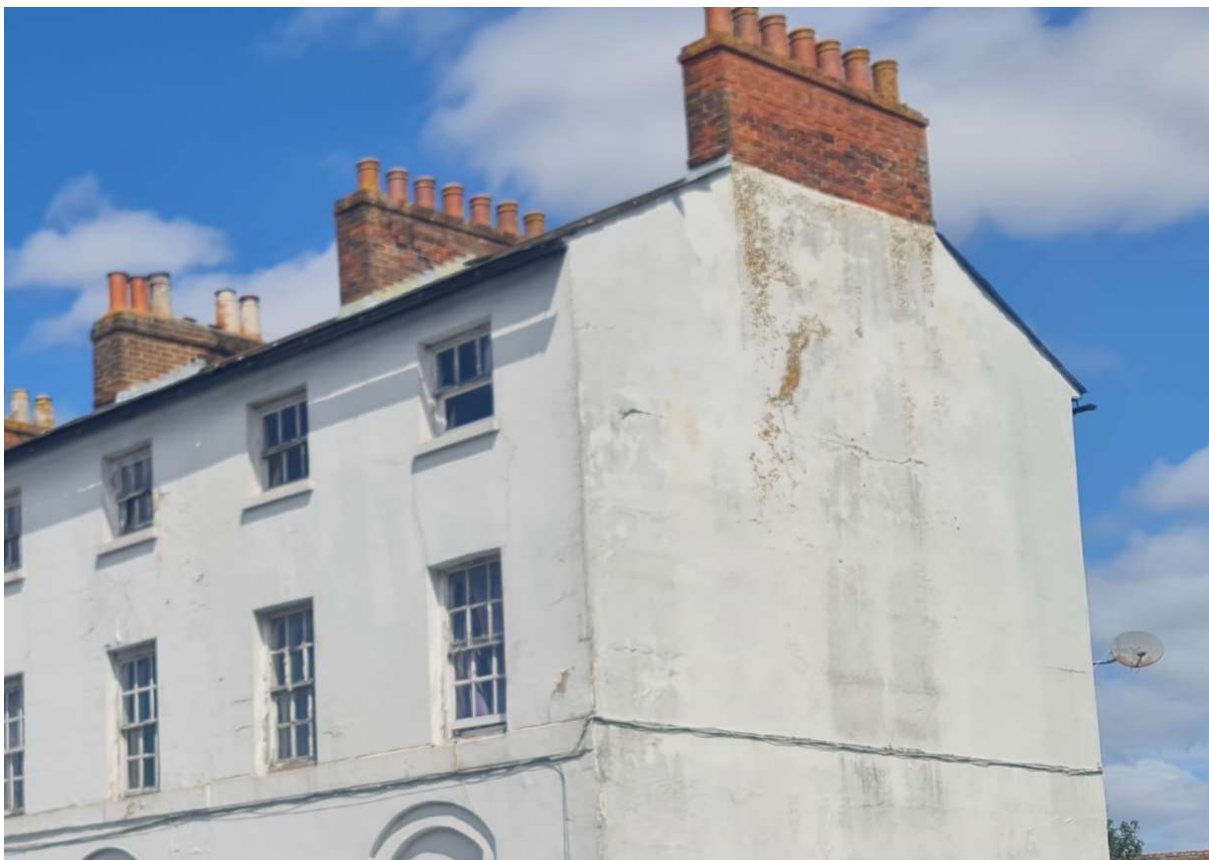
Figure 5: Detailed photos of flank elevation showing poor state of stucco
