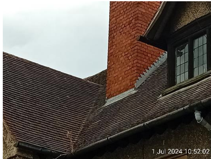
Figure 24: Example of tight lead flashing around chimney.
