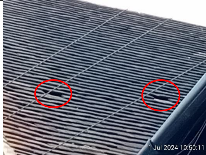
Figure 20: Example of missing tiles.
