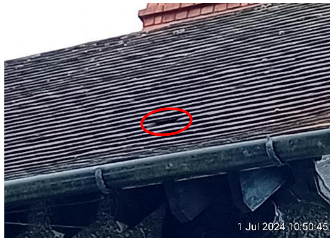
Figure 21: Example of missing roof tile.
