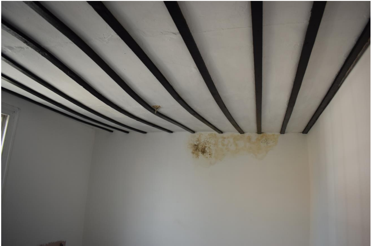
Plate 8 sagging first-floor ceiling
