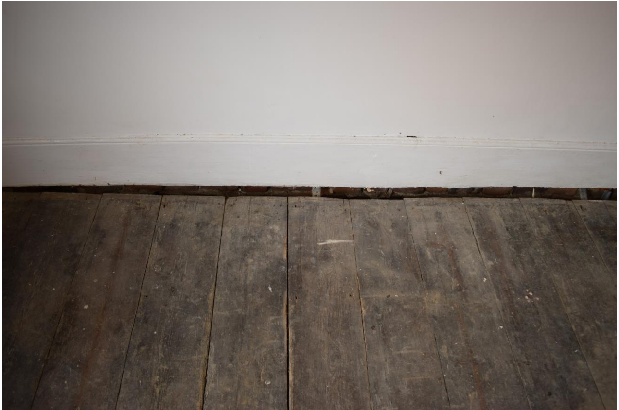
Plate 12 gap between wall and floor on the first floor
