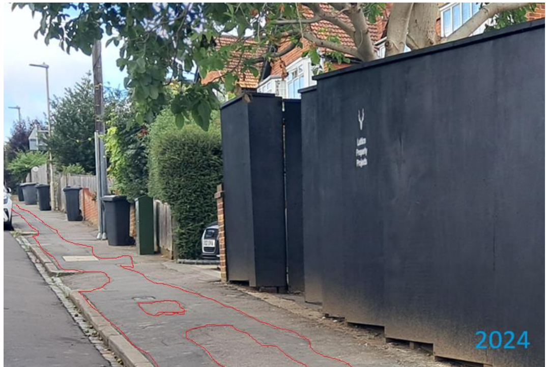
Images 9-11 – Dated images showing additional service trenches within the rooting area of T001 (Walnut)
