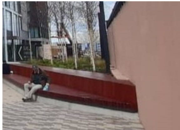
Rear wall to planter on right next to boundary wall to be made good
