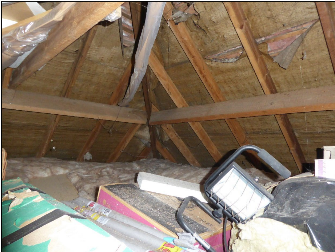
Figure 11. Example loft space and torn tar paper. 1 Briar Close, Caversham. 31.07.24
