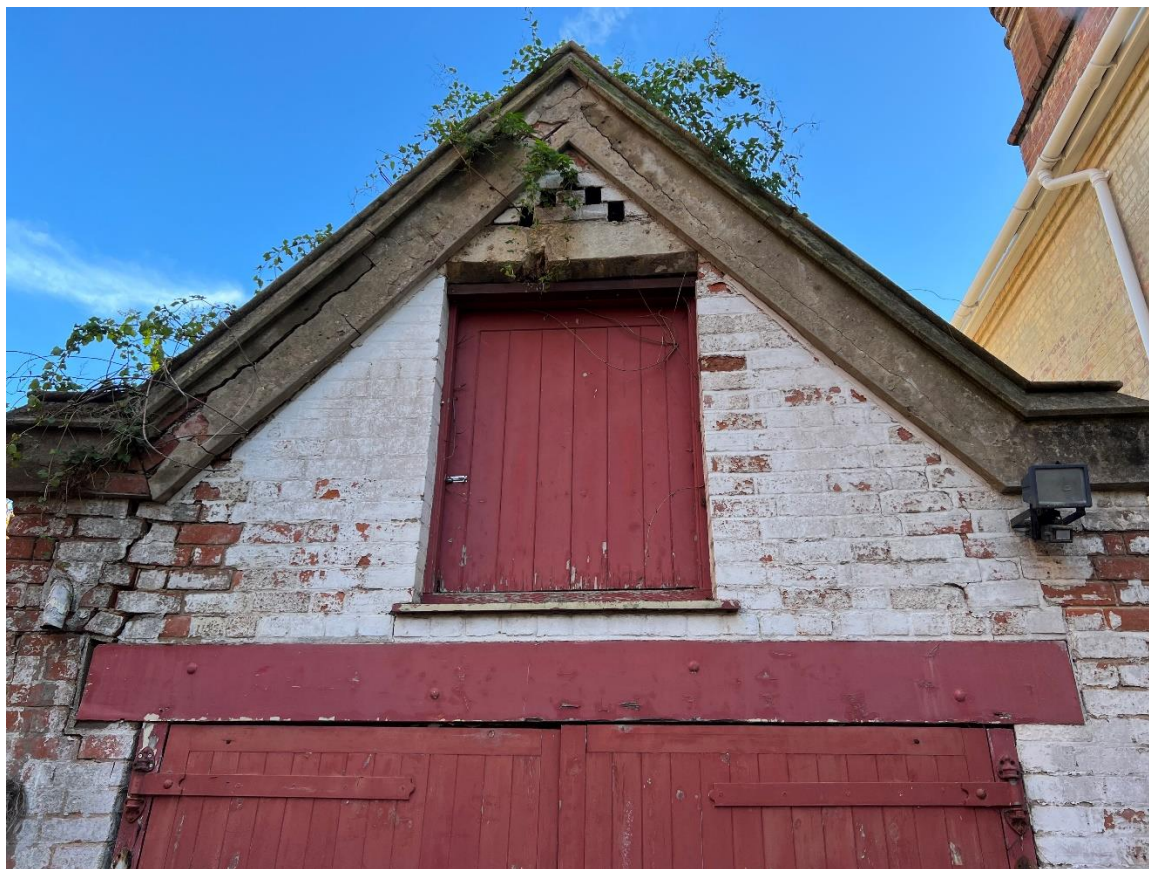
The west façade of the garage showing cracking to the north side
