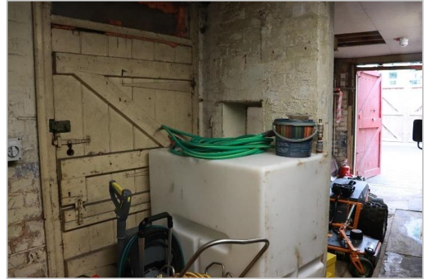
Interior view of side access door
