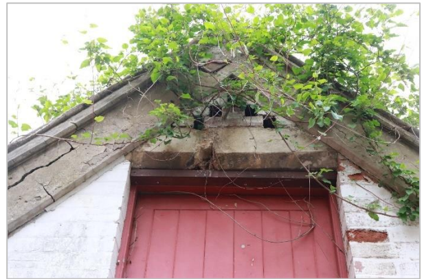
Western Elevation detail – ventilation design, sandstone lintel, vegetation growth and render fracture
