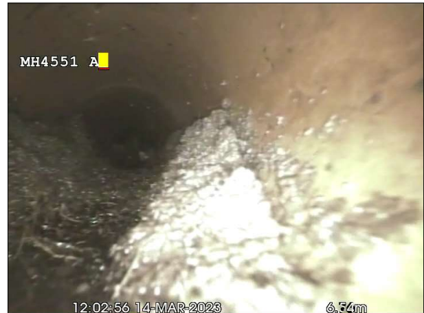
Photo: 10_4b, 00:00:00 6.5m, Debris silt, 30 % cross-sectional area loss, Start
