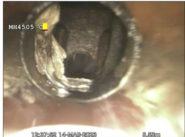
Photo: 54_6a, 00:00:00 8.5m, Debris grease, from 06 to 11 o'clock, 30 % cross-sectional area loss
