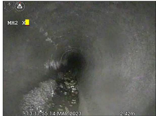
Photo: 28_3b, 00:00:00 0.1m, Debris silt, 10 % cross-sectional area loss, Start
