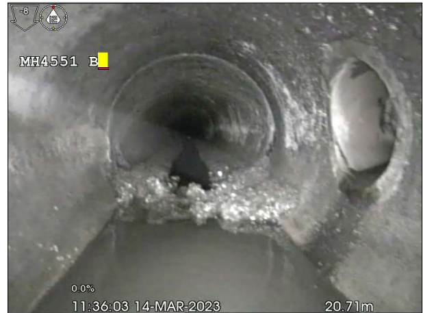
Photo: 86_10a, 00:00:00 20.6m, Debris silt, 10 % cross-sectional area loss, Finish
