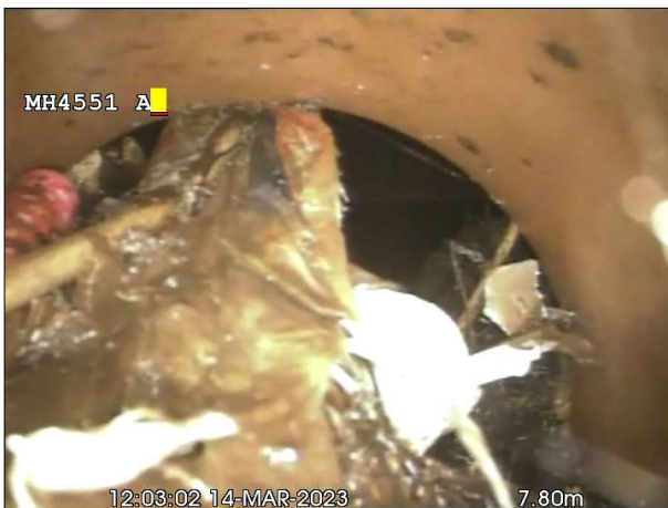
Photo: 10_5a, 00:00:00 7.8m, Debris silt, 80 % cross-sectional area loss, Finish
