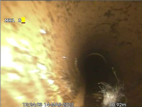
Photo: 11_4a, 00:00:00 11m, Debris, 5 % cross-sectional area loss
