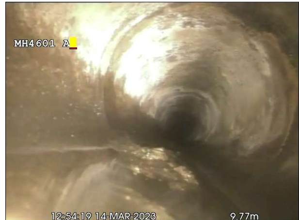
Photo: 92_6a, 00:00:00 9.8m, Debris silt, 10 % cross-sectional area loss, Finish
