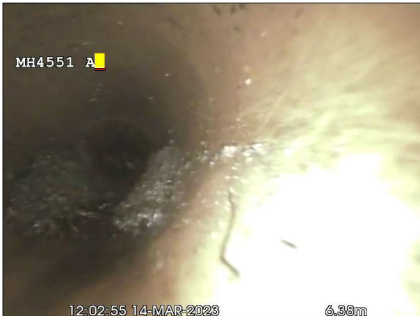
Photo: 10_4a, 00:00:00 6.5m, Debris silt, 30 % cross-sectional area loss, Start
