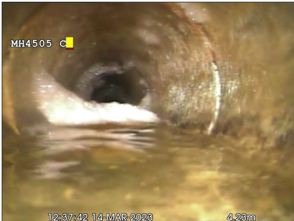
Photo: 53_5a, 00:00:00 4.3m, Debris grease, from 05 to 08 o'clock, 15 % cross-sectional area loss
