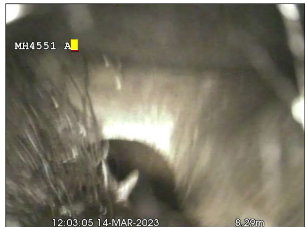
Photo: 10_7a, 00:00:00 8.3m, Debris silt, 20 % cross-sectional area loss
