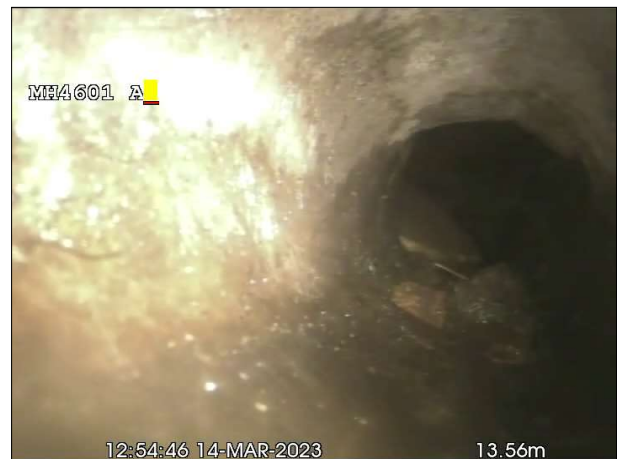
Photo: 93_7b, 00:00:00 13.5m, Debris, 15 % cross-sectional area loss
