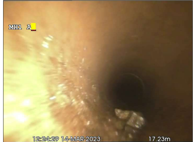
Photo: 12_5a, 00:00:00 17.5m, Debris, 10 % cross-sectional area loss
