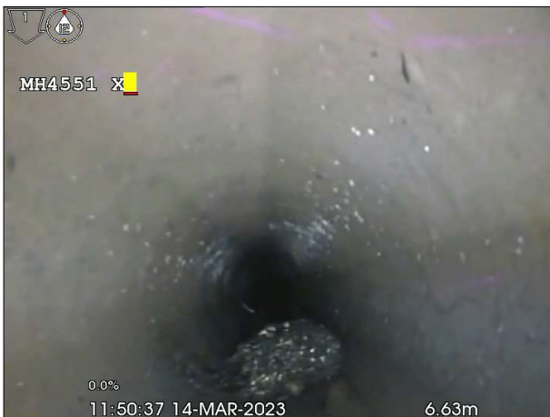
Photo: 61_6a, 00:00:00 7m, Debris silt, 15 % cross-sectional area loss
