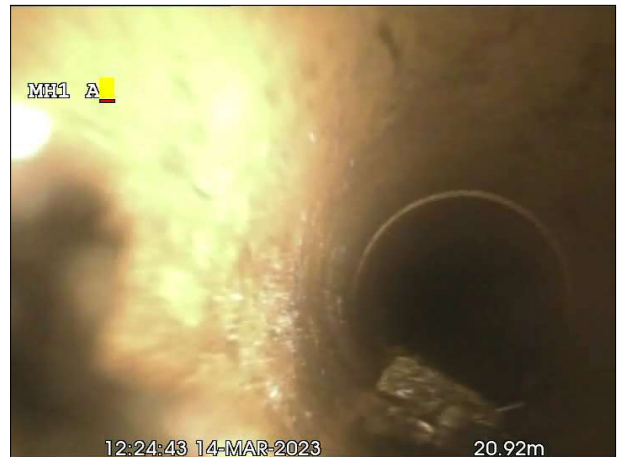
Photo: 14_7a, 00:00:00 21.7m, Debris, 15 % cross-sectional area loss
