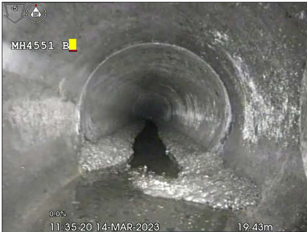
Photo: 84_9a, 00:00:00 20m, Debris silt, 10 % cross-sectional area loss, Start
