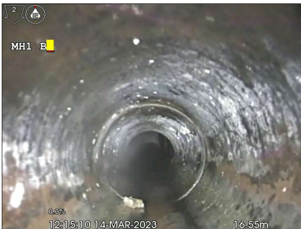
Photo: 23_6a, 00:00:00 16.7m, Debris, 5 % cross-sectional area loss
