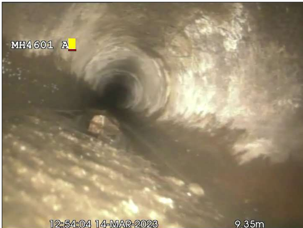
Photo: 91_5a, 00:00:00 9.3m, Debris silt, 10 % cross-sectional area loss, Start
