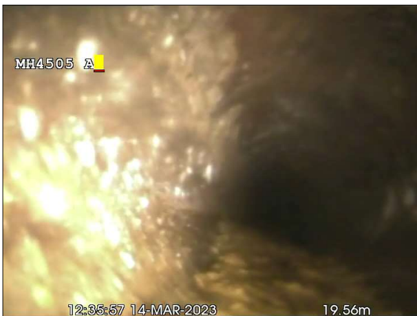
Photo: 41_9a, 00:00:00 19.5m, Debris grease, from 05 to 07 o'clock, 10 % cross-sectional area loss, Start
