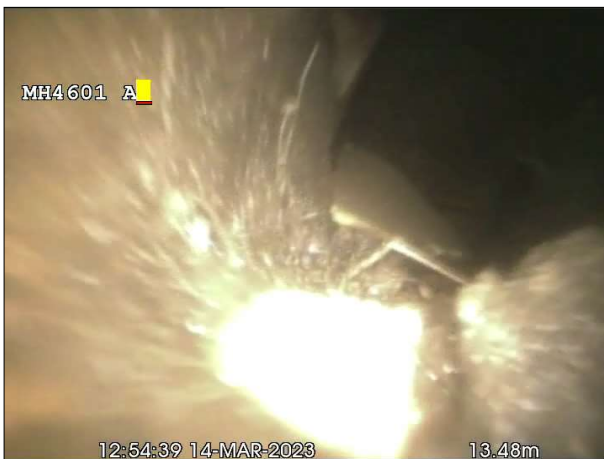
Photo: 93_7a, 00:00:00 13.5m, Debris, 15 % cross-sectional area loss
