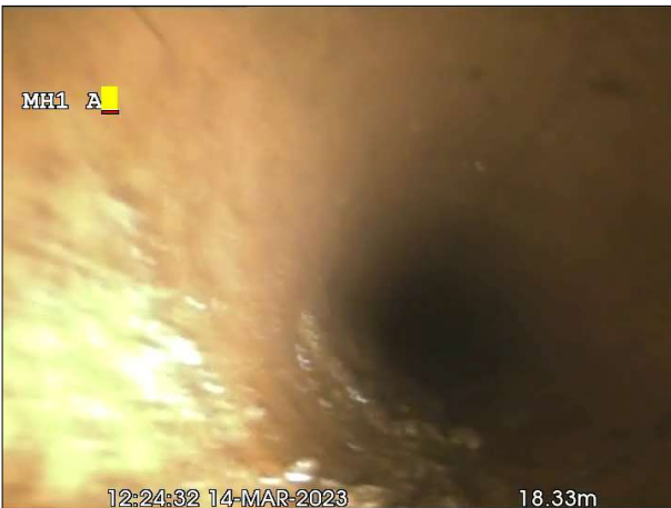
Photo: 13_6a, 00:00:00 18.2m, Debris silt, 5 % cross-sectional area loss, Start
