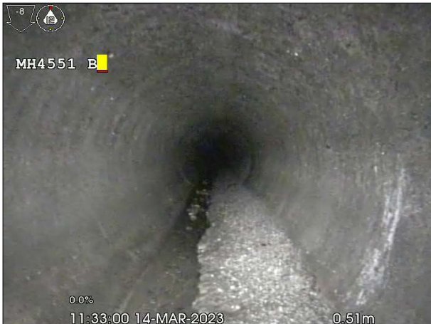
Photo: 78_3a, 00:00:00 0.2m, Debris silt, 10 % cross-sectional area loss, Start
