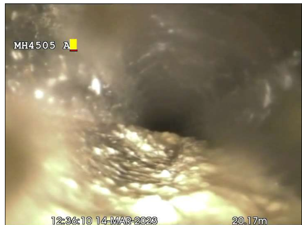
Photo: 43_10a, 00:00:00 20.3m, Debris grease, from 05 to 07 o'clock, 20 % cross-sectional area loss, Finish
