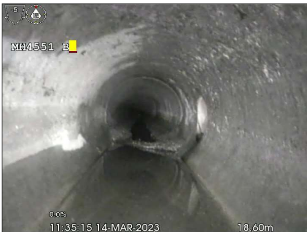
Photo: 82_7a, 00:00:00 18.6m, Debris silt, 0 % cross-sectional area loss, Finish
