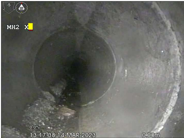
Photo: 28_3a, 00:00:00 0.1m, Debris silt, 10 % cross-sectional area loss, Start
