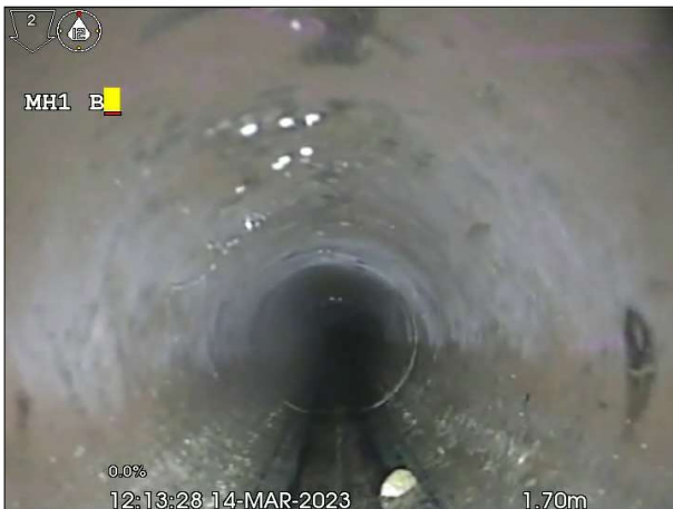
Photo: 21_4a, 00:00:00 1.8m, Debris, 5 % cross-sectional area loss
