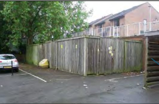
Generator, AST and substation compound on western boundary
