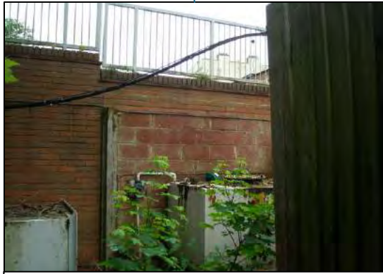
AST and fuel line
