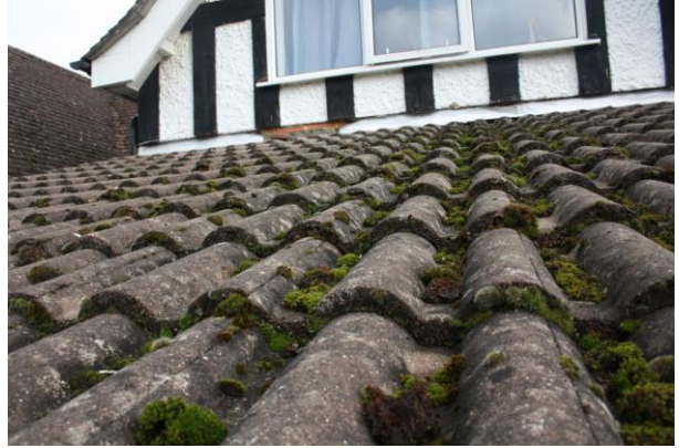
Photo 4: Mossy roof tiles
