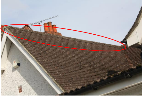
Photo 3: Concrete roof tiles with localised gaps under ridge
