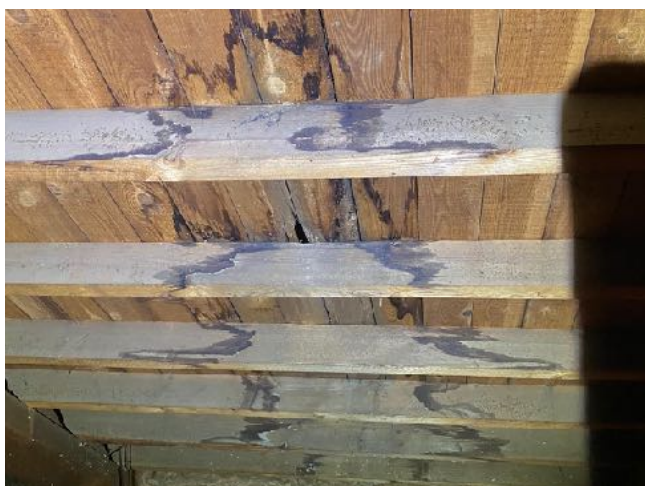
Image 9: Water stained wooden panelling.
