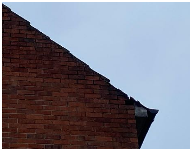
Image 4: Missing brick on eastern gable end
