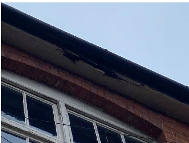
Image 5: Rotting soffit box from water damage on northern elevation
