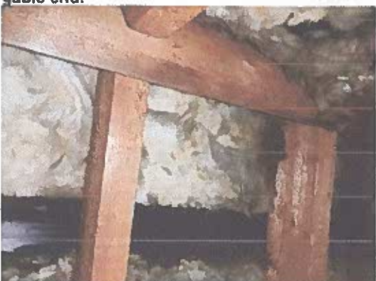
7. Plastic roofing felt behind fibreglass insulation.
