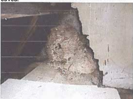
5. Large hornet's nest at the southwestern gable end.
