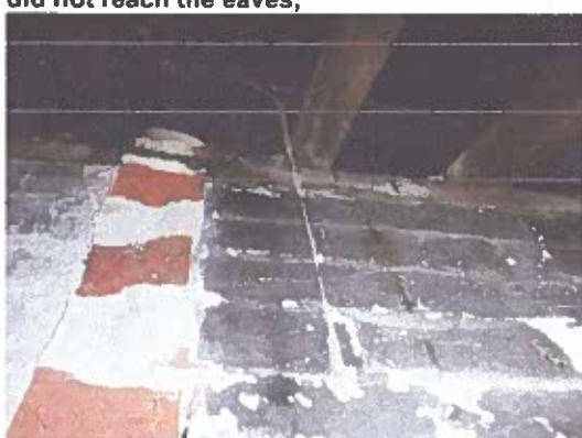
14. Daylight and roof tiles visible along the ridge.
