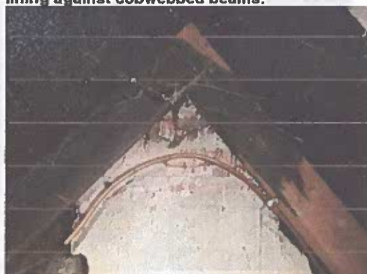
4. Slight gap between timbers and breezeblock gable.
