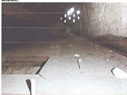
12. Fibreglass insulation under boarding which did not reach the eaves,
