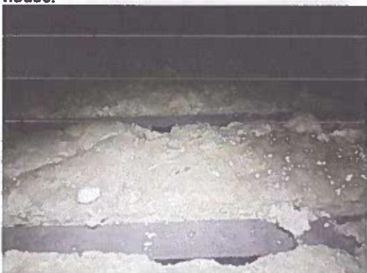
3. Fibreglass insulation that was tight to the eaves.
