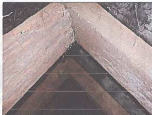
2. Mostly intact bitumen and hessian felt roof lining against cobwebbed beams.
