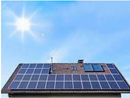
Figure 6: Photovoltaic (PV) Panels
