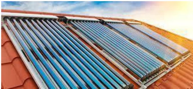
Figure 4: Solar Thermal Panels
