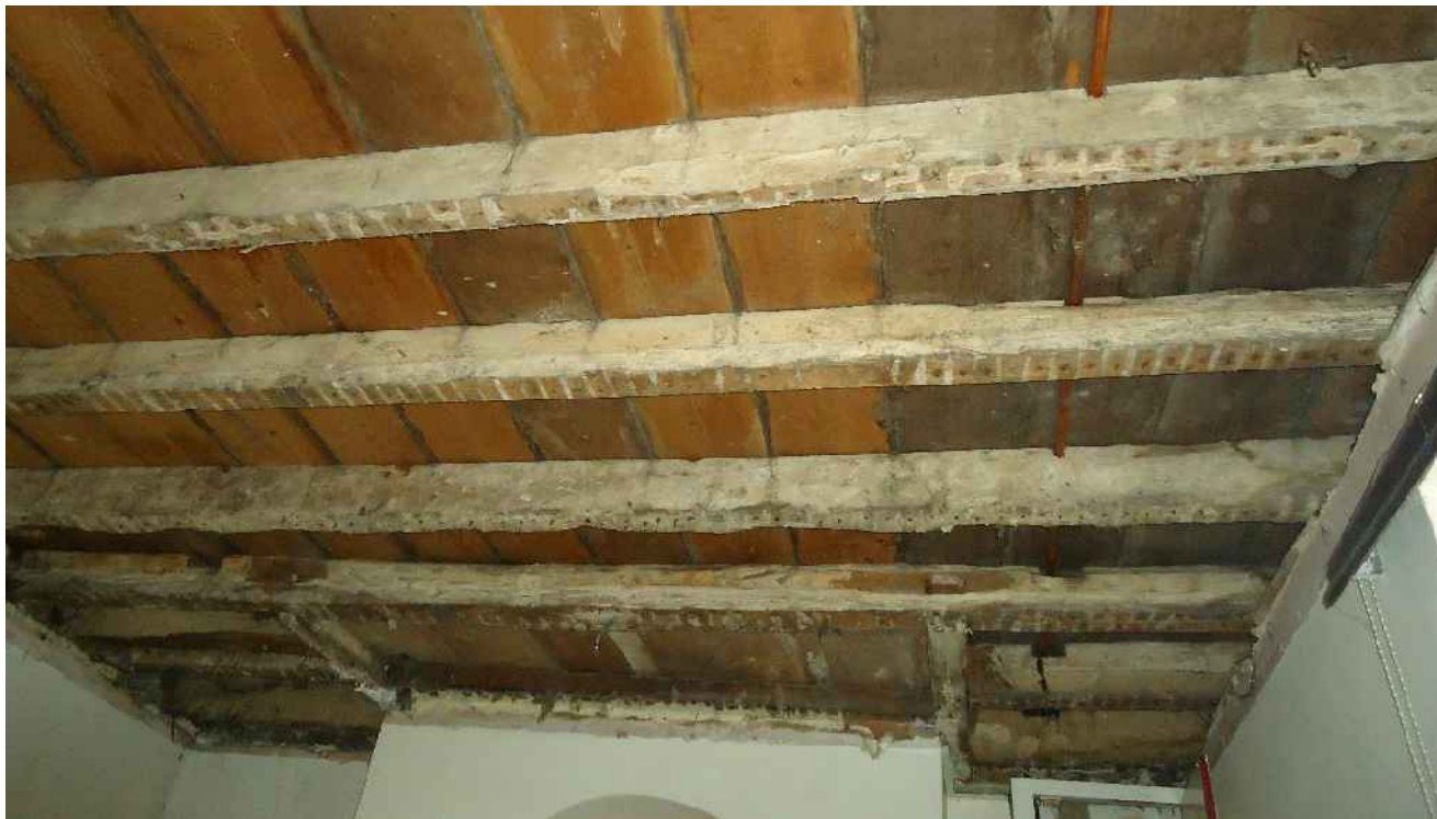
Living/ Bedroom Ceiling Joists rotten and having damp issues See drawing A-1005
