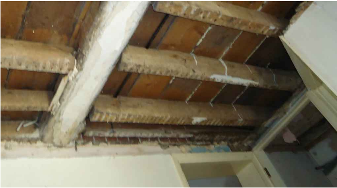
Kitchen/Bathroom Issues with ceiling joists and beam not being adequate and damp to joists. See drawing A-1005
