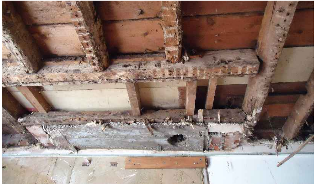
kitchen Rotten Ceiling Joist with damp issues. See drawing A-1005
