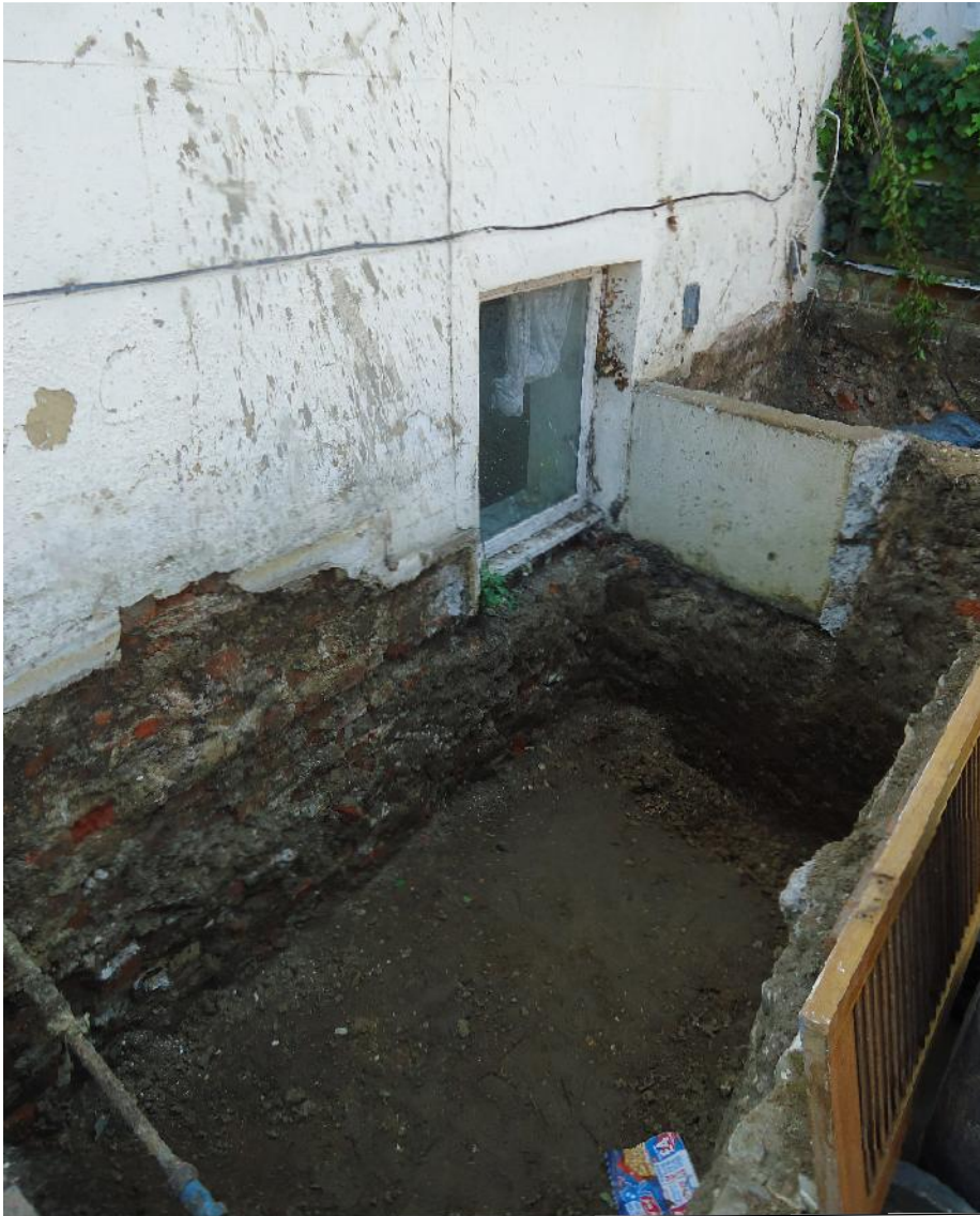
Living Front Wall, water and damp issues See drawing A-1005
