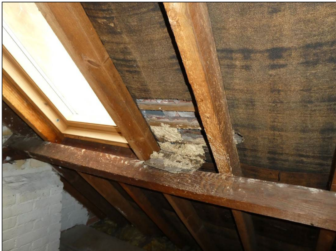
Figure 13. Example of ripped bitumen lining in loft. 8 Avebury Square, Reading. 13.02.24
