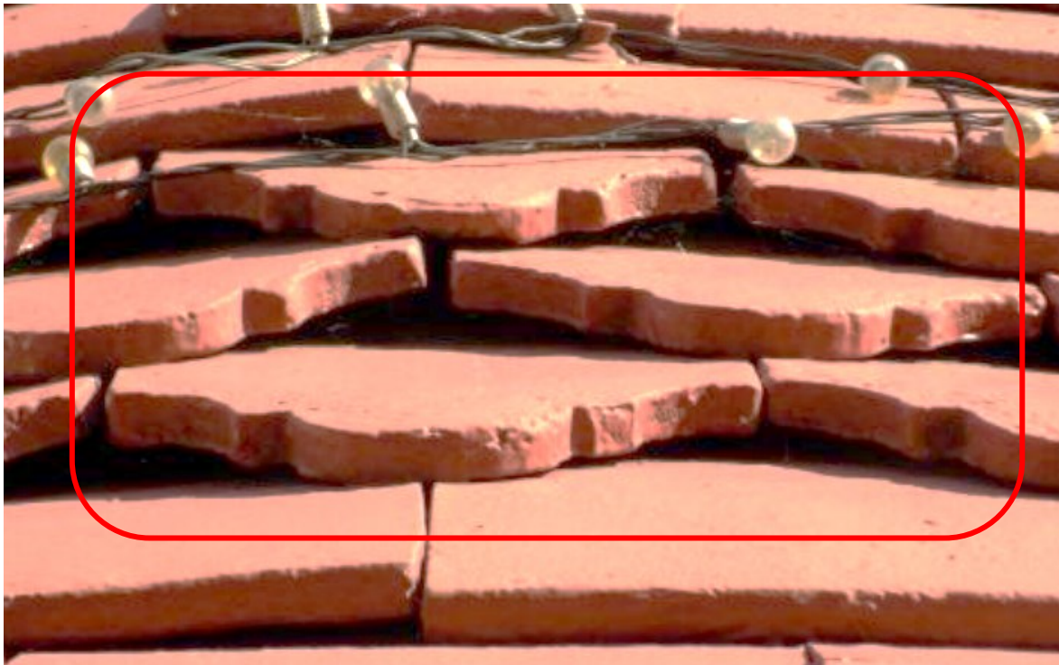
Image 3 – Vertical hanging tiles within the front elevation which look to offer shelter opportunities of value to crevice dwelling species
