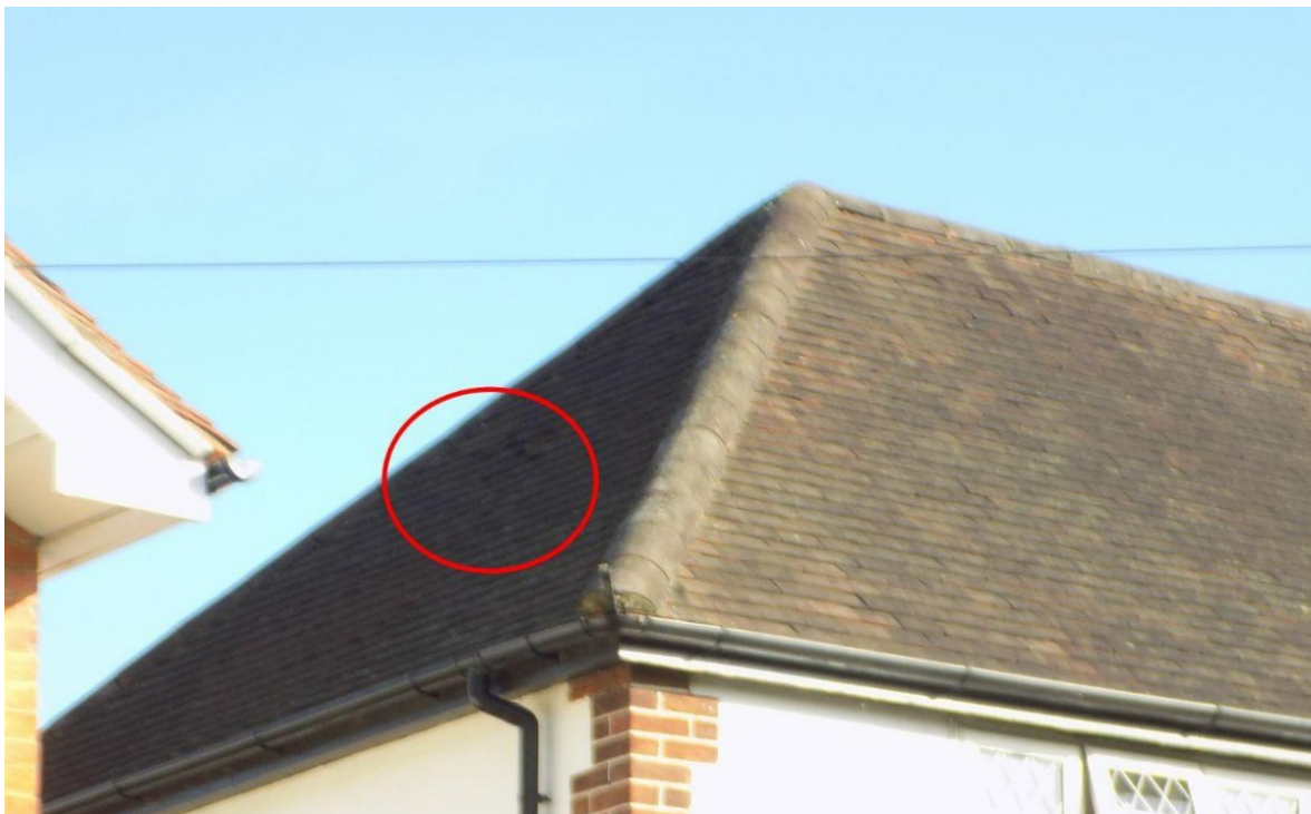
Image 6 – North/West facing elevation of the property offering further gaps of value within the roof coverings
