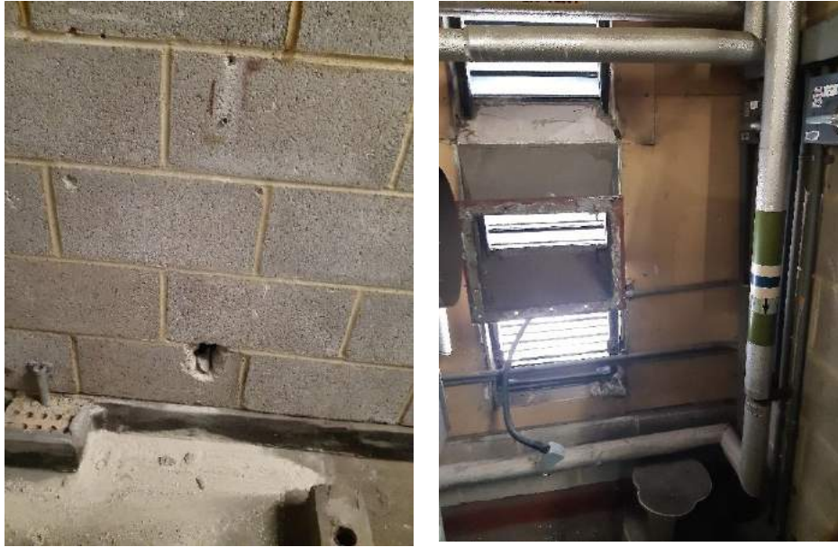
Image 8 (left): Hole in mortar in breezeblock wall in B3. Image 9 (right): Light ingress through vents
