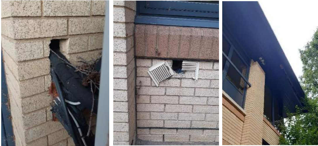
Image 3 (left): Cables coming out of wall on B2. Image 4 (middle): Broken vent on B2. Image 5 (right): Missing soffit box panels on B3.
