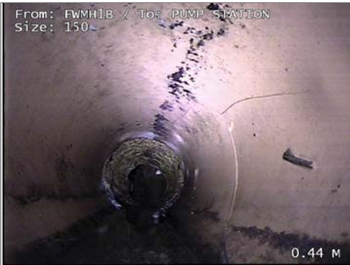
Cracks multiple from 1 to 5 o'clock
