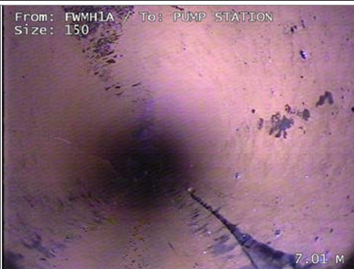
Crack longitudinal at 9 o'clock, Start
