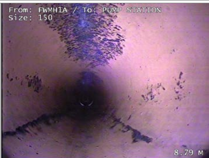
Crack longitudinal at 9 o'clock, Start, Finished
