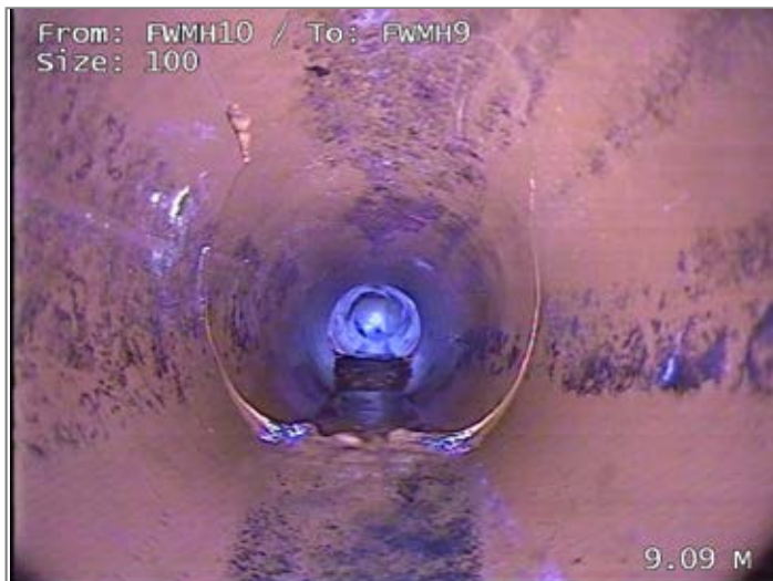
Crack circumferential from 1 to 11 o'clock
