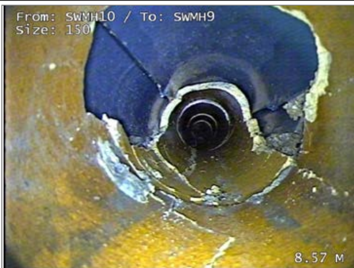
Broken pipe from 8 to 4 o'clock
