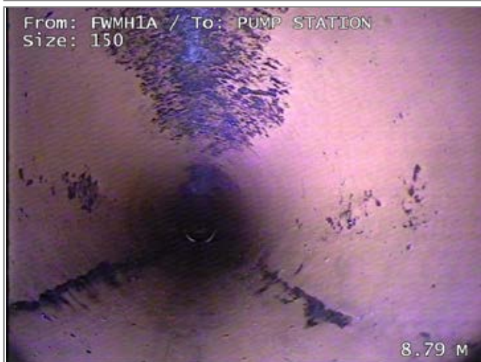
Crack longitudinal at 5 o'clock, Start, Finished
