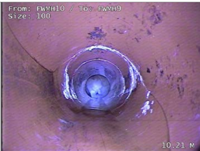
Cracks multiple from 9 to 5 o'clock
