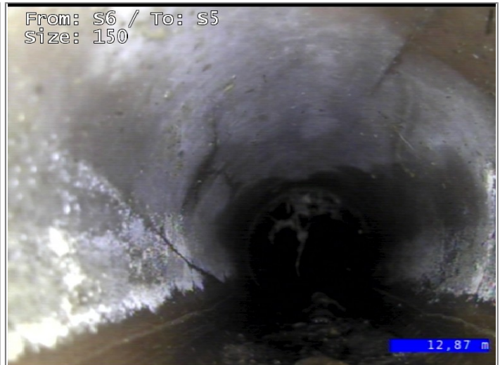
Crack longitudinal at 9 o'clock
