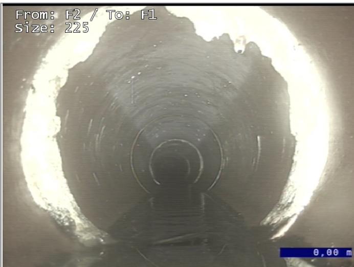
Attached deposits, encrustation from 7 to 5 o'clock 10% cross-sectional area loss
