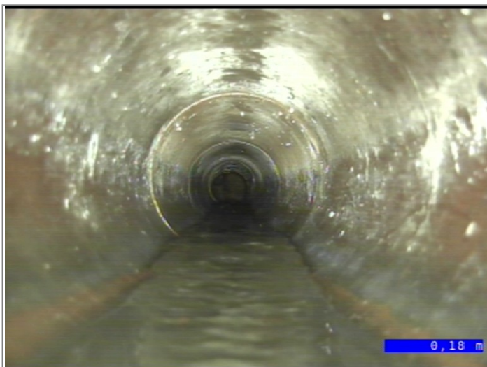
Start node type, manhole, reference F2
