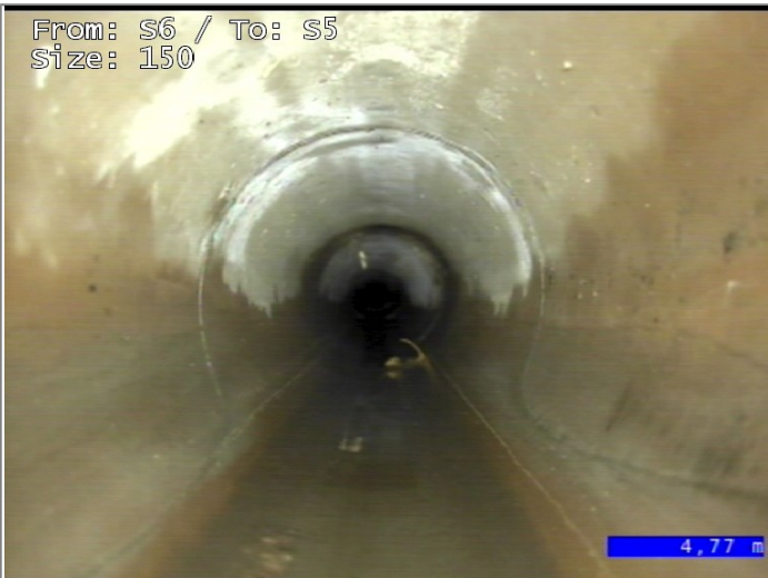
Crack circumferential from 8 to 4 o'clock
