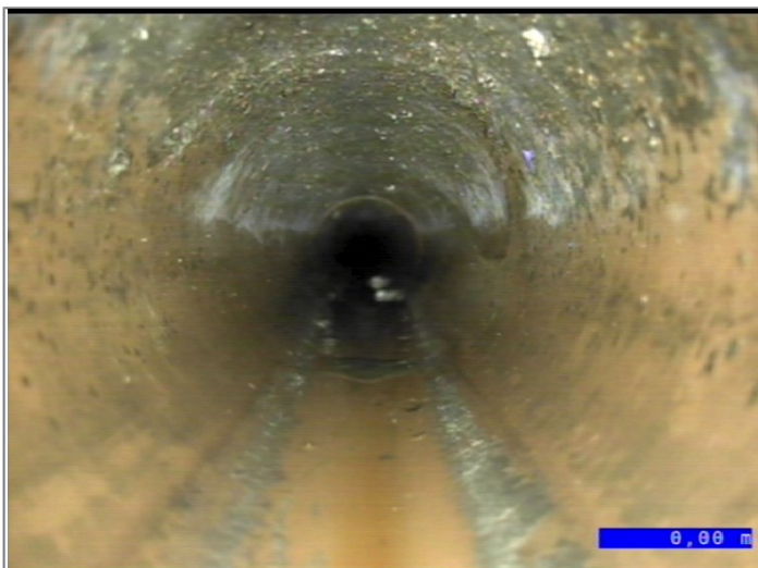
Start node type, manhole, reference F5
