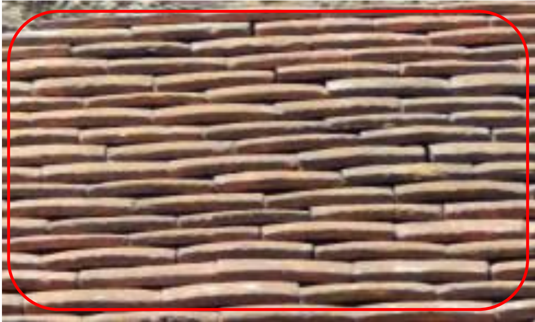
Image 7 – Further gaps of value to bats observed within the rear North elevation of the property from the shape of the tile
