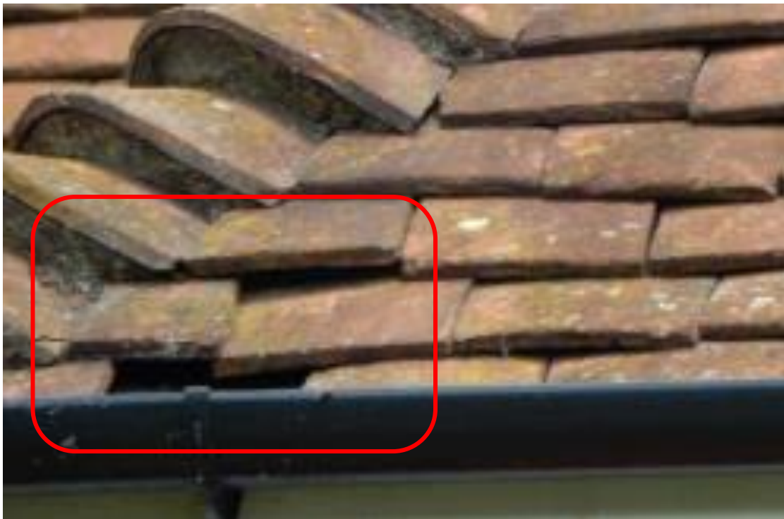
Image 4 – Further gaps of value to bats observed within the rear West elevation of the property
