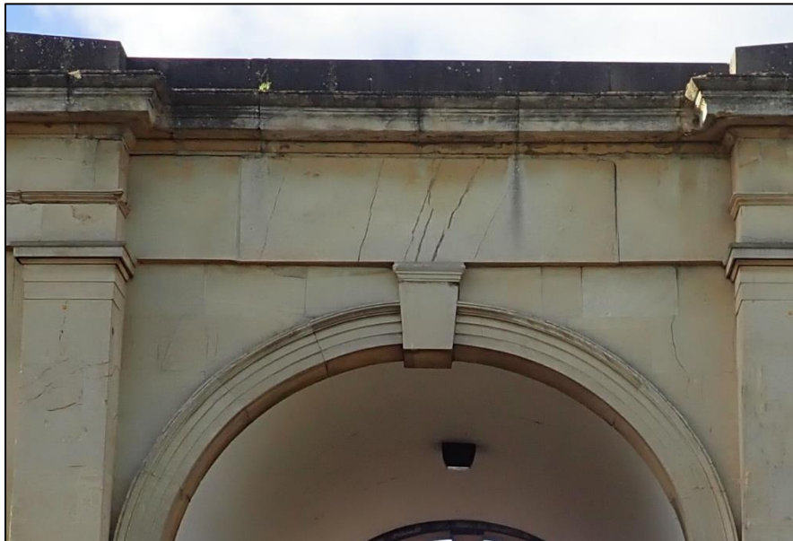
Figure 25. Diagonal cracks in the architrave over the keystone.
