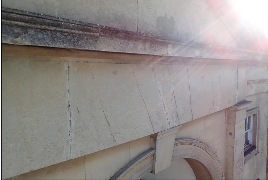
Figure 13. Near-vertical cracks and open joints in the architrave.
