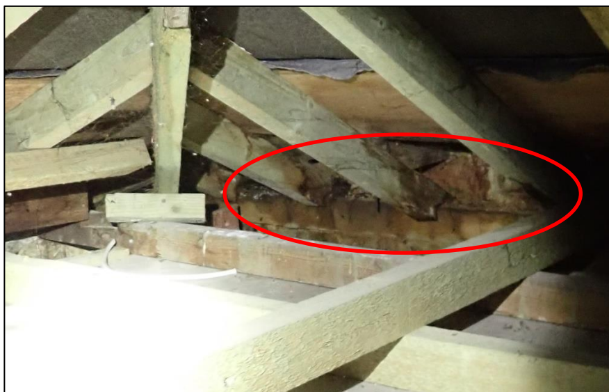
Figure 46. Possible water ingress at the southern end of the west elevation.
