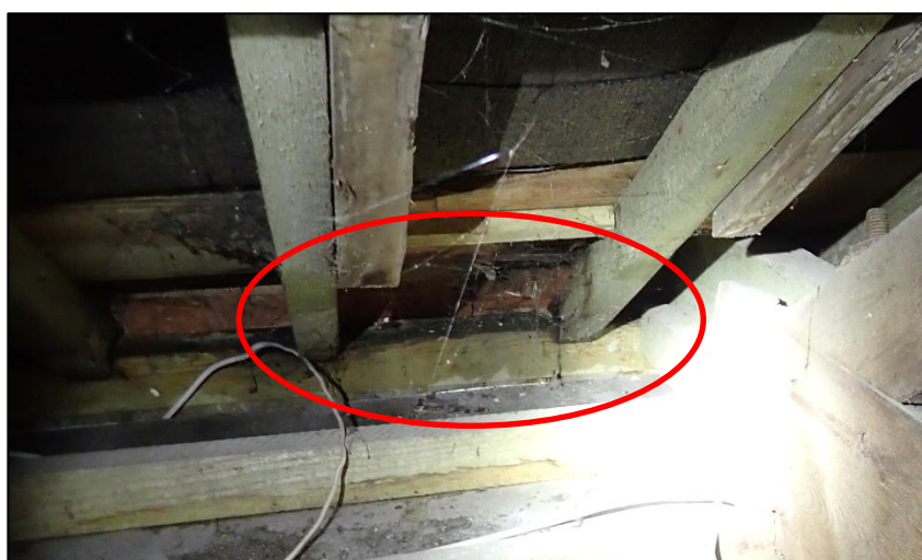
Figure 45. Possible water ingress on the east side of the roof/to the north of the northern truss.
