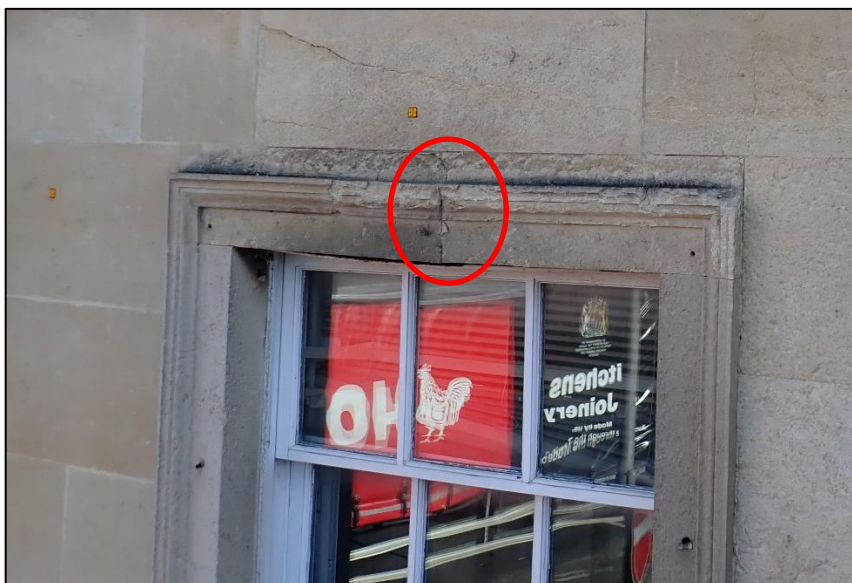
Figure 14. Very slight, vertical crack in the stone lintel.
