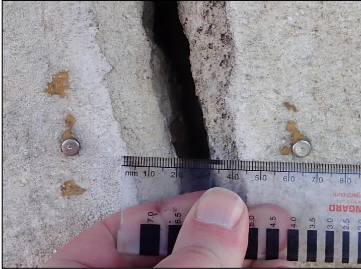
Figure 7. Close-up view of the crack at the Demec Studs.
