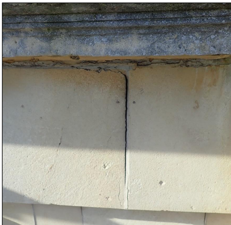
Figure 21. Tapered crack/open joint in the frieze to the north of the keystone.
