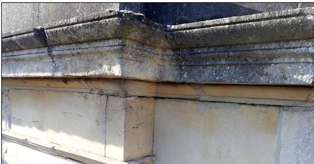
Figure 23. Horizontal gap in the mortar below the cornice.
