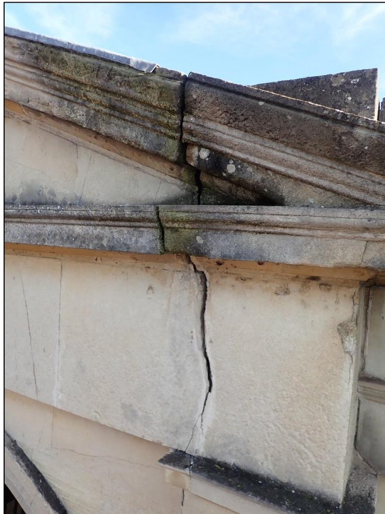
Figure 6. Tapered crack at the southern end of the architrave over the archway.
