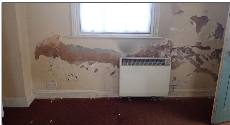
Figure 47. Example of blistering in the plaster and paint.
