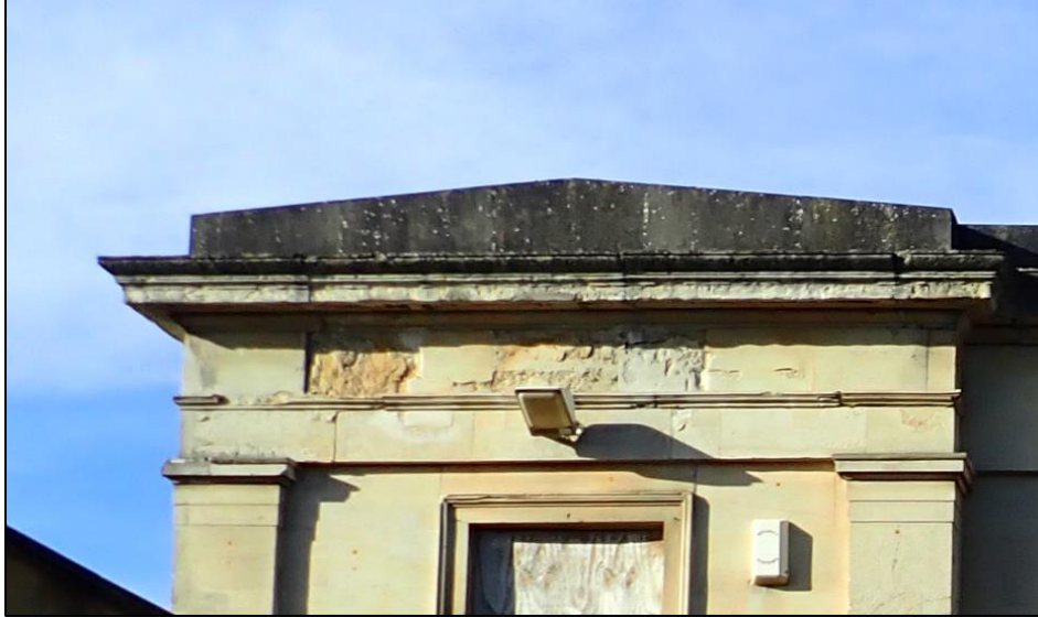
Figure 24. Erosion in the frieze on the south lodge.
