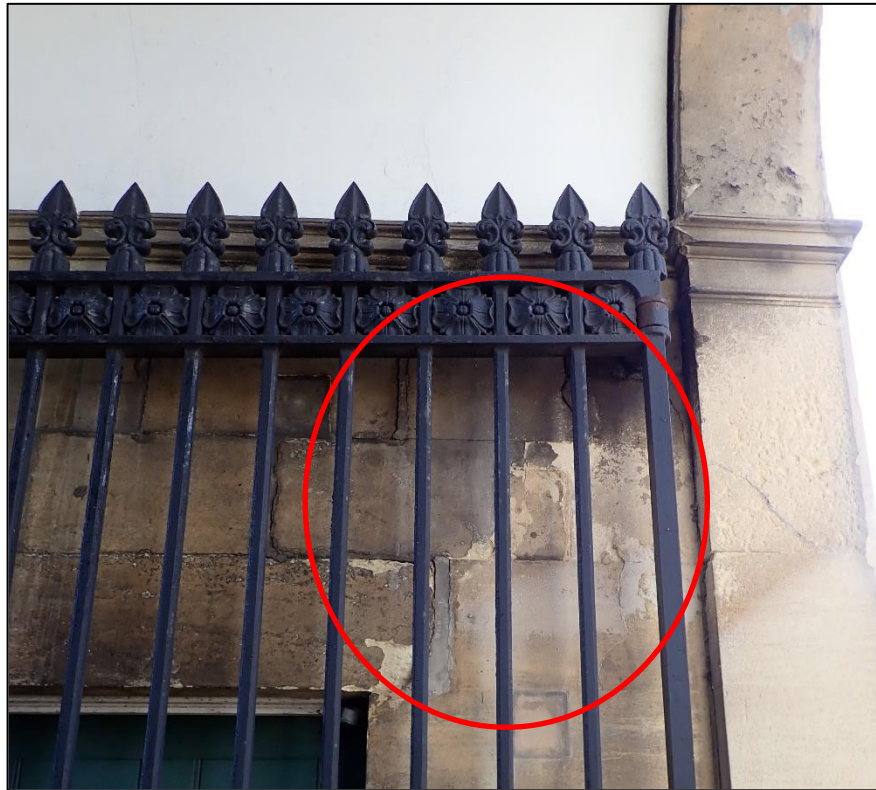
Figure 39. Stepped crack/scar between the door and the arch.
