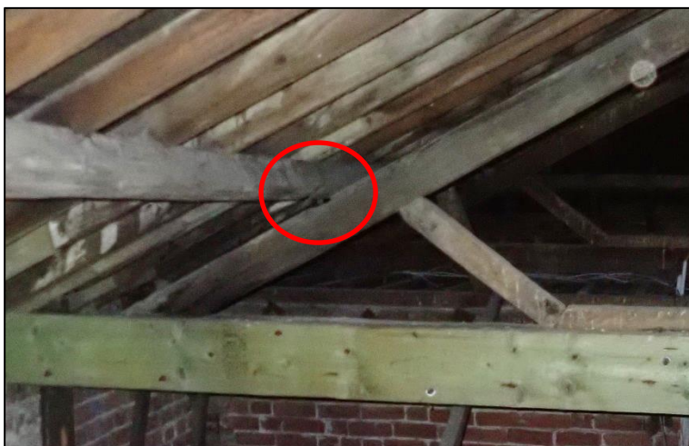
Figure 44. View of the gap between the underside of the rear purlin and the principal rafter.
