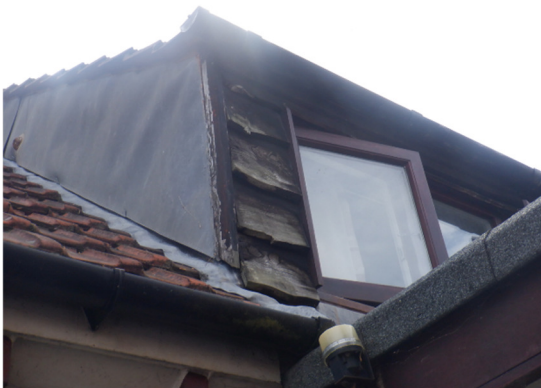
9. Lifted waney edge timbers on the dormer window, viewed from the northeast.
