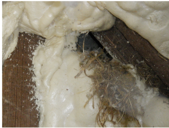
20. Large gap within eastern gable with bird nesting material.
