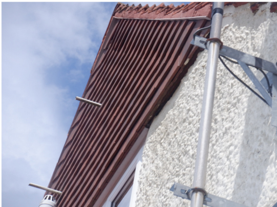
11. Occasionally lifted hanging tiles on the rear gable, viewed from the southwest.
