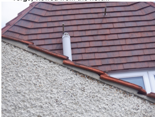
6. Crumbling verge mortar, viewed from the west.
