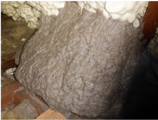
19. Large wasp nest situated at the base of the chimney.
