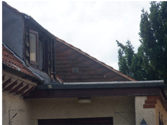
12. Occasionally lifted hanging tiles on the eastern gable of the existing side extension, viewed from the east.
