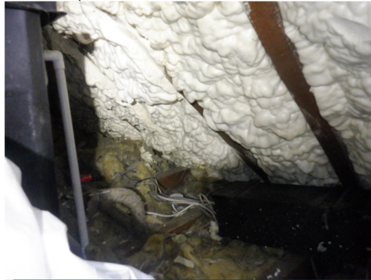
16. Roof void heavily insulated with expanding foam over bitumen felt.
