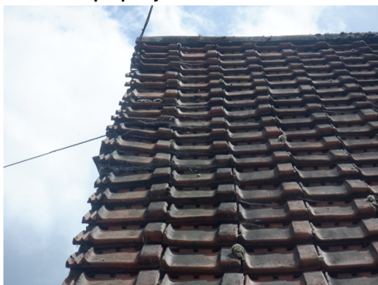
4. Lifted interlocking roof tiles along the front verge, viewed from the north.
