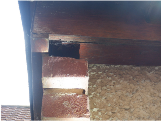
13. Damaged timber soffit, viewed from the north.
