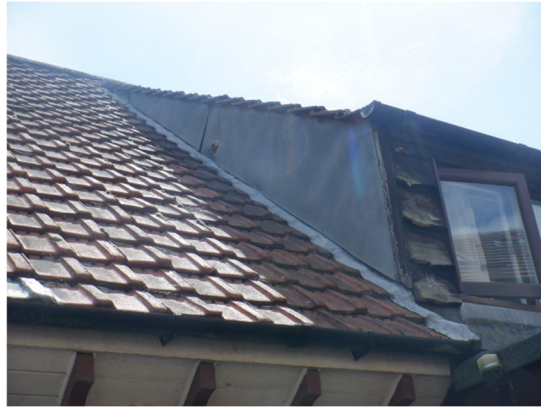
8. Slight gaps between lead flashing and dormer window, viewed from the north.
