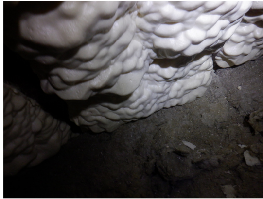
18. Eaves blocked by expanding foam.
