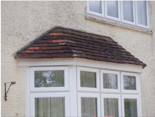
15. Occasionally lifted clay roof tiles on the front bay window, viewed from the southeast.
