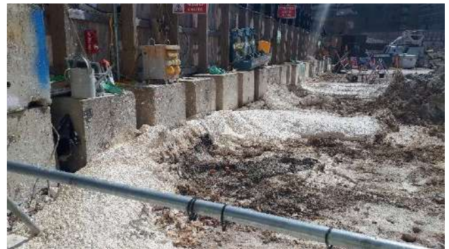
Photo 8 – A close-up view of an installed pile on the northern boundary of the site. A sludge material can be seen on the ground surface.
