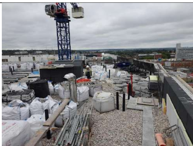
Photo 11 – Fire damage on Level 12 of Block E.
