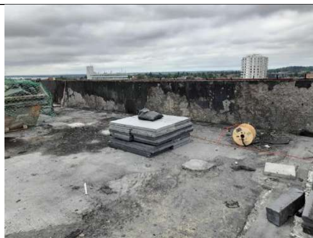
Photo 12 – Fire damage on Level 12 of Block E.
