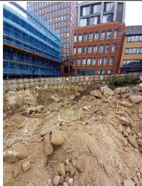
Photo 6 – View of broken out concrete slabs and exposed Made Ground in the northeast of site.
