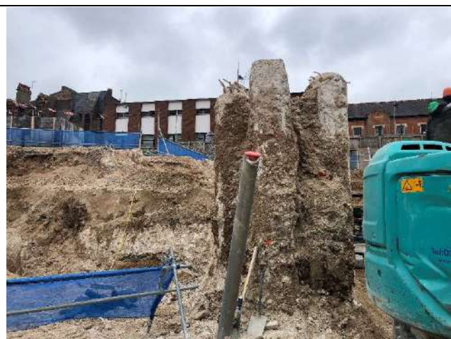
Photo 2 – Exposed piles within southwest of the site.
