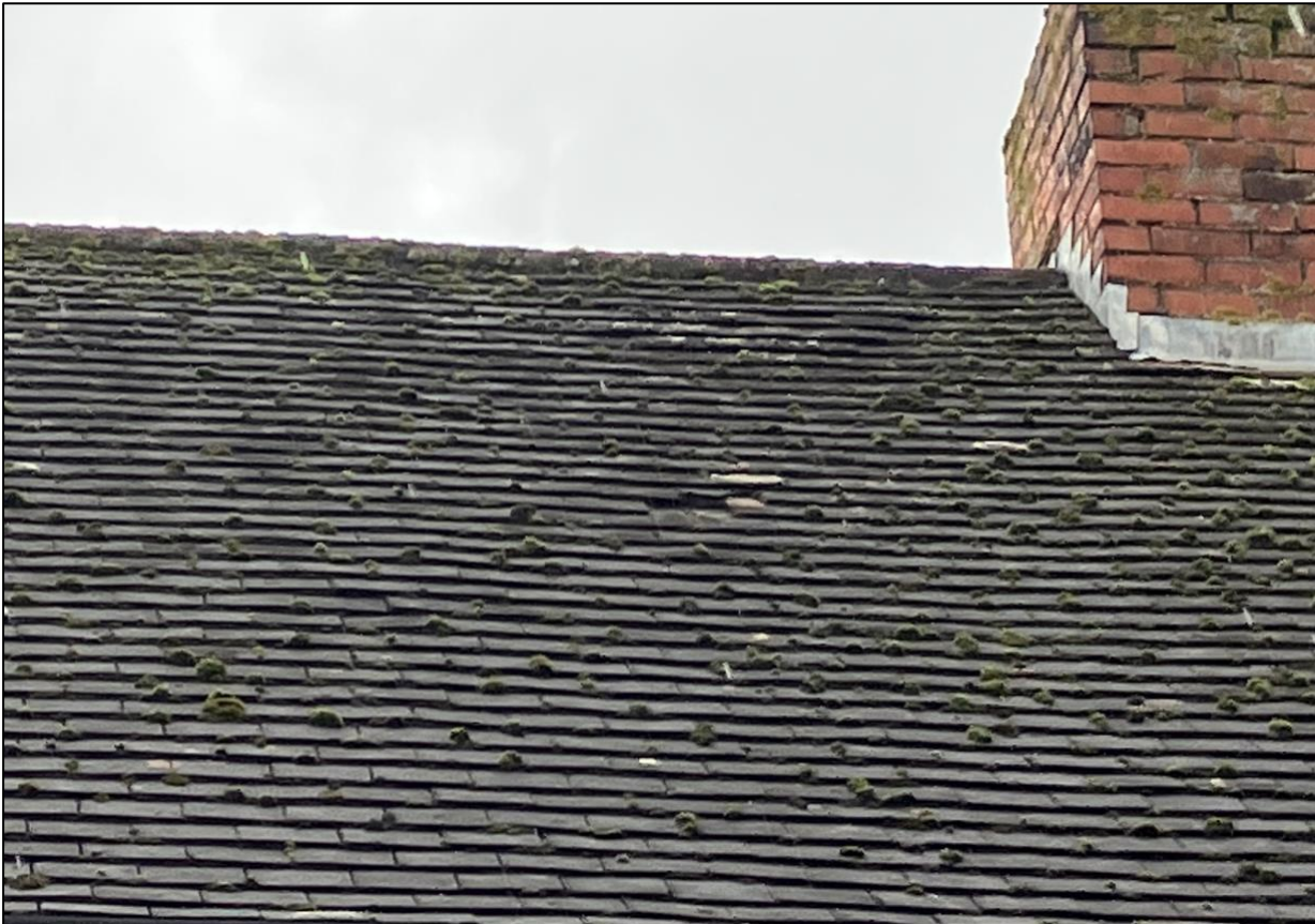
Photograph 3. The one broken tile observed on the north-eastern aspect of the dwelling's roof.
