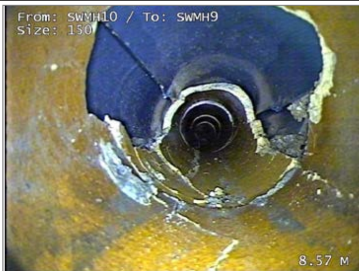
Broken pipe from 8 to 4 o'clock
