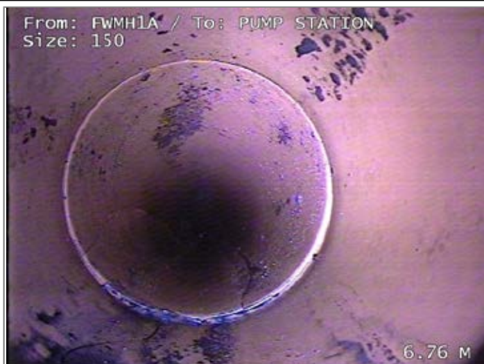
Crack longitudinal at 5 o'clock, Start
