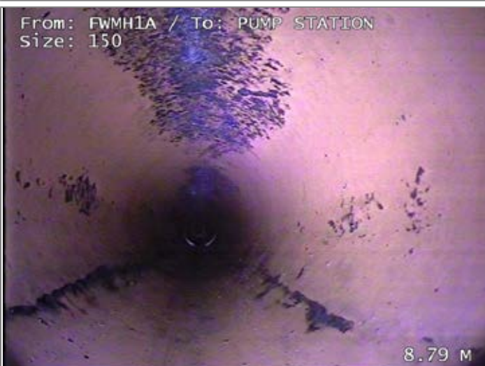
Crack longitudinal at 9 o'clock, Start, Finished
