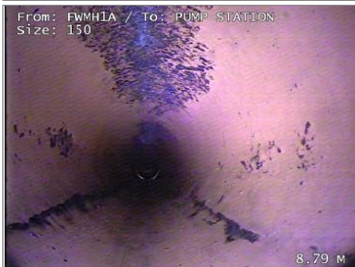
Crack longitudinal at 5 o'clock, Start, Finished
