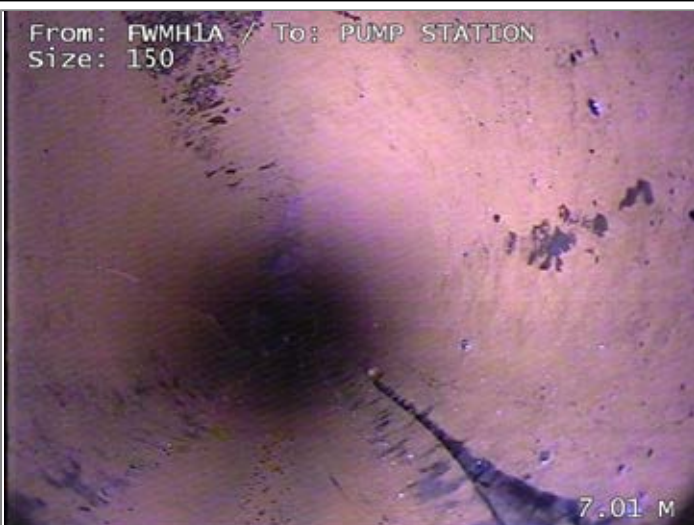
Crack longitudinal at 9 o'clock, Start
