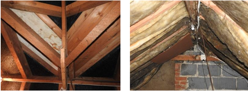
Figs. 24 & 25 Cobwebbed plumb cut and gable end
