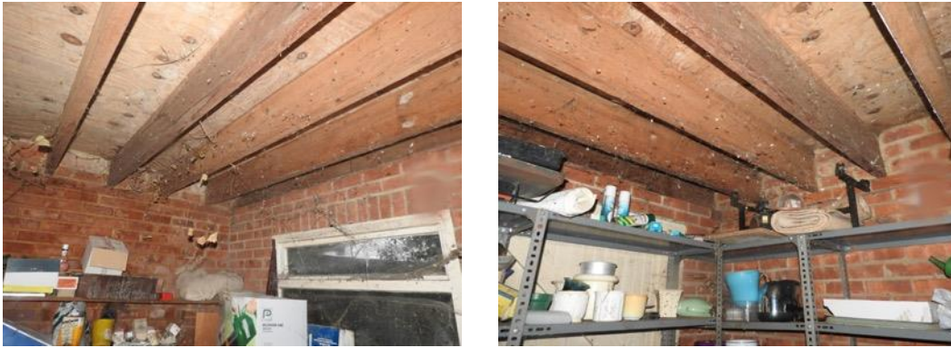
Figs. 29 & 30 Cobwebbed garage roof
