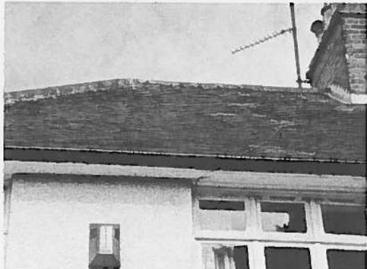
6. Slight gaps within clay roofing tiles
