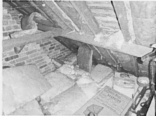
14. Fibreglass insulation throughout the roof space.
